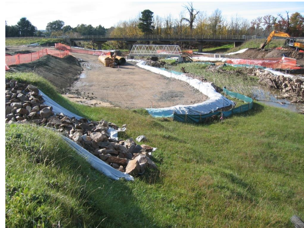
FIGURE 2: EXAMPLE OF A CONSTRUCTION PAD WITH RAISED CONTAINMENT BUND AROUND PERIPHERY (MUCH LARGER THAN PROPOSED FOR THIS SITE)
