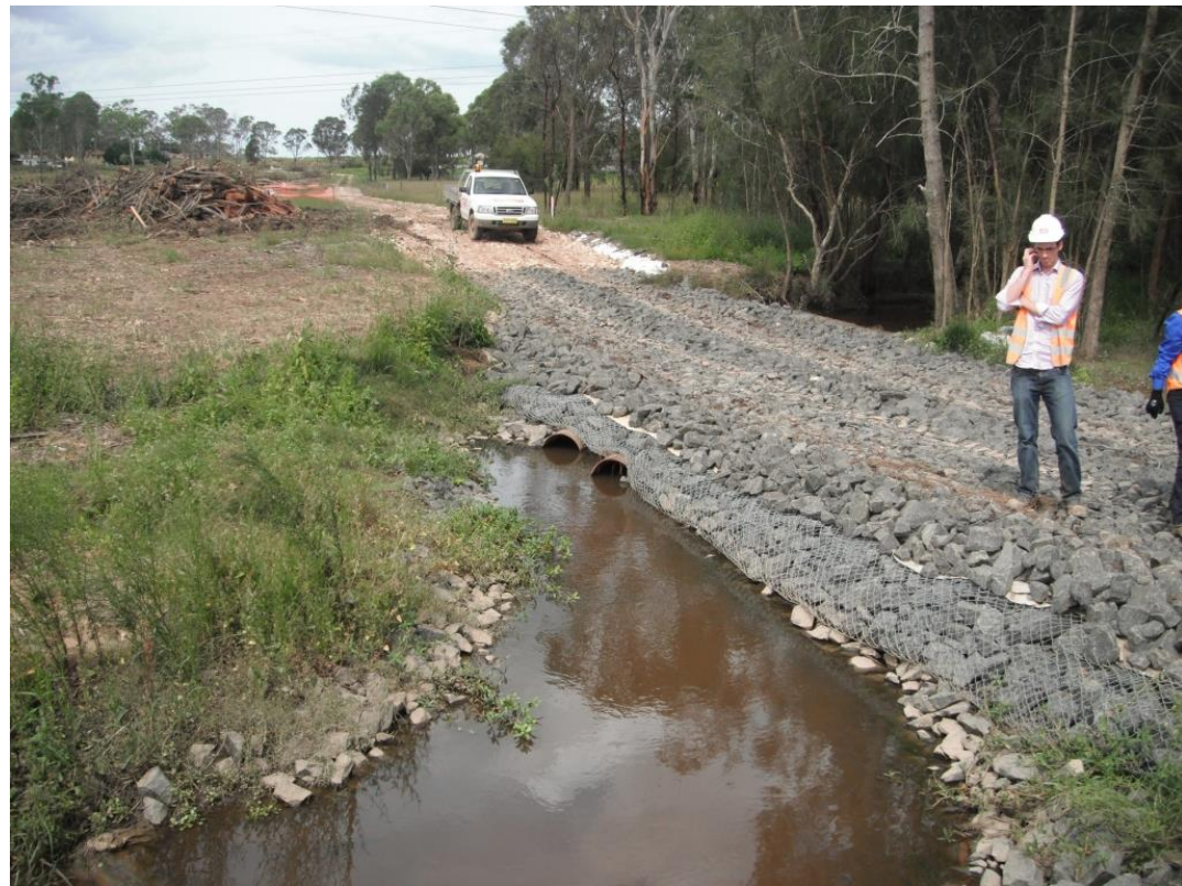
FIGURE 1: EXAMPLE OF GOOD QUALITY CLEAN, DURABLE ROCK USED AS A CONSTRUCTION PAD/ACCESS IN A WATERCOURSE
