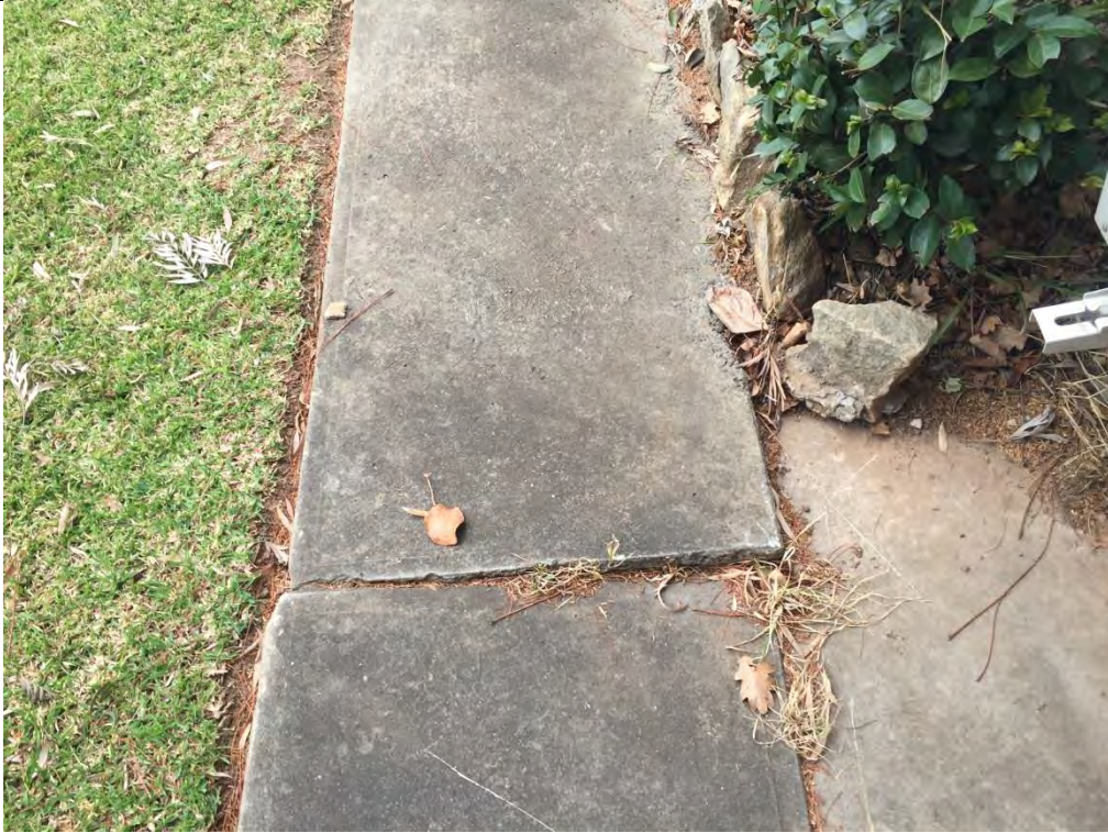
Photo 17 – Cracks in concrete caused by subsidence
