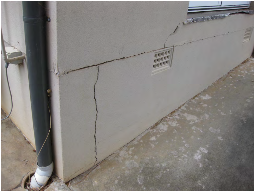
Photo 4 - Damage to Acquired House in Tahmoor Court, Tahmoor
