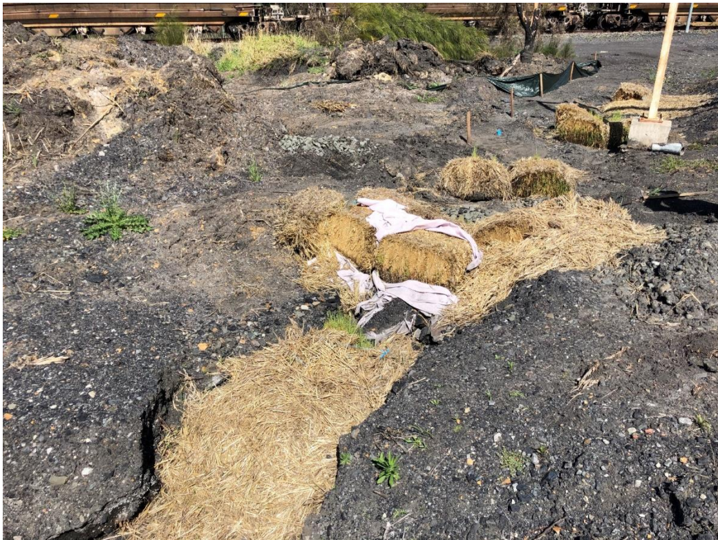
Photo 25 Erosion in batters adjacent to LDP1. Repair recommended
