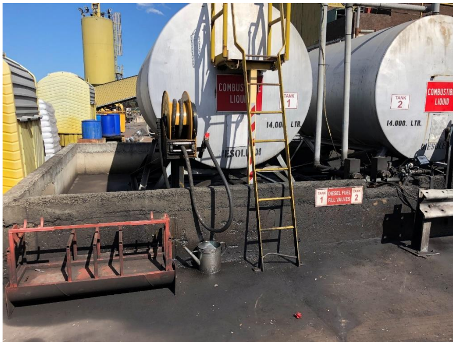
Photo 4 Appropriate bunding of diesel fuel area. However, some hydrocarbon staining evident. Recommend clean up
