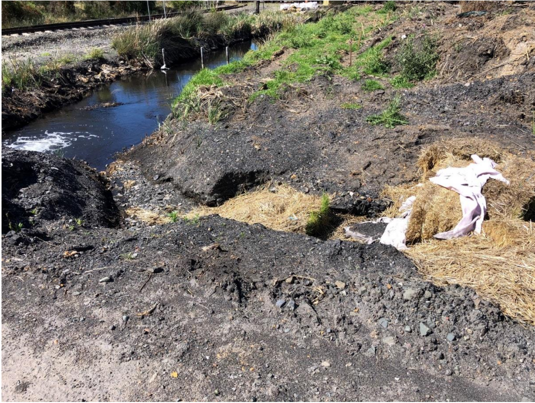
Photo 24 Erosion in batters adjacent to LDP1. Repair recommended
