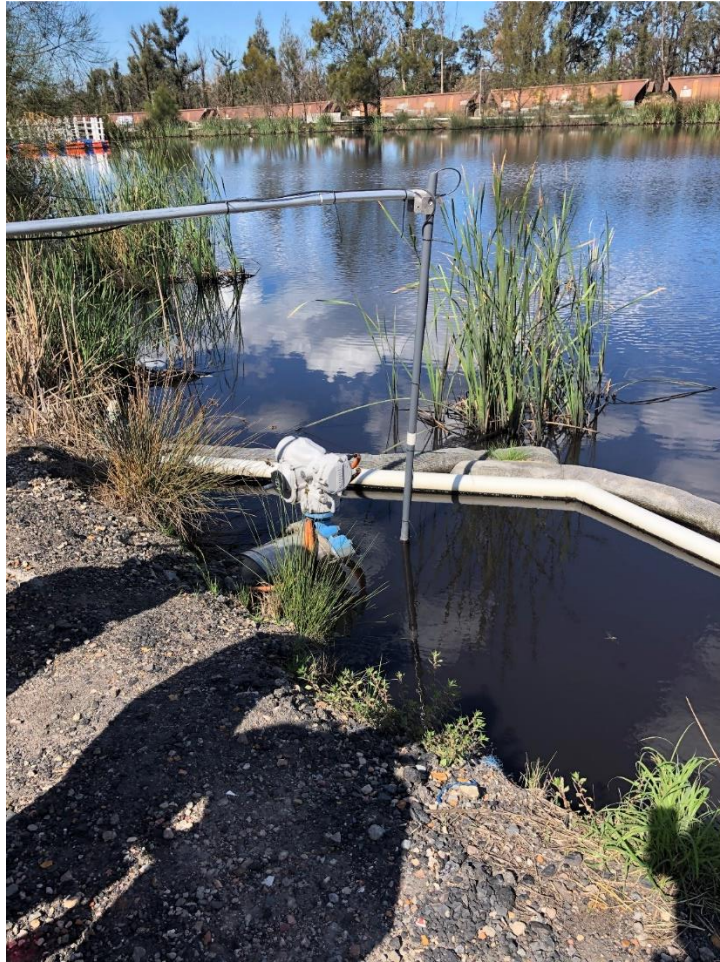
Photo 3 Real time turbidity monitor installed in M4 following April 2020 incident
