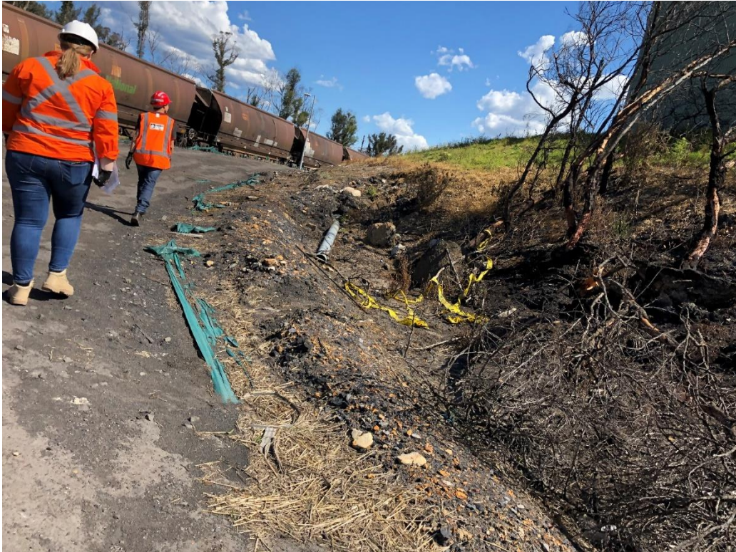
Photo 26 Erosion between Water Treatment Plant and LDP1 following damage to sediment controls in bushfires. Repair recommended
