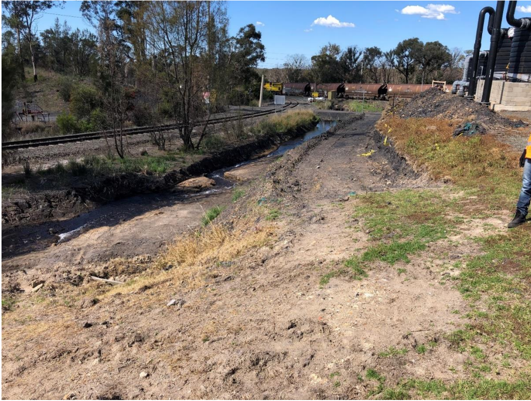
Photo 1 Cleanout works between Dam M4 and LDP 1. Erosion and sediment controls recommended prior to revegetation and stabilisation
