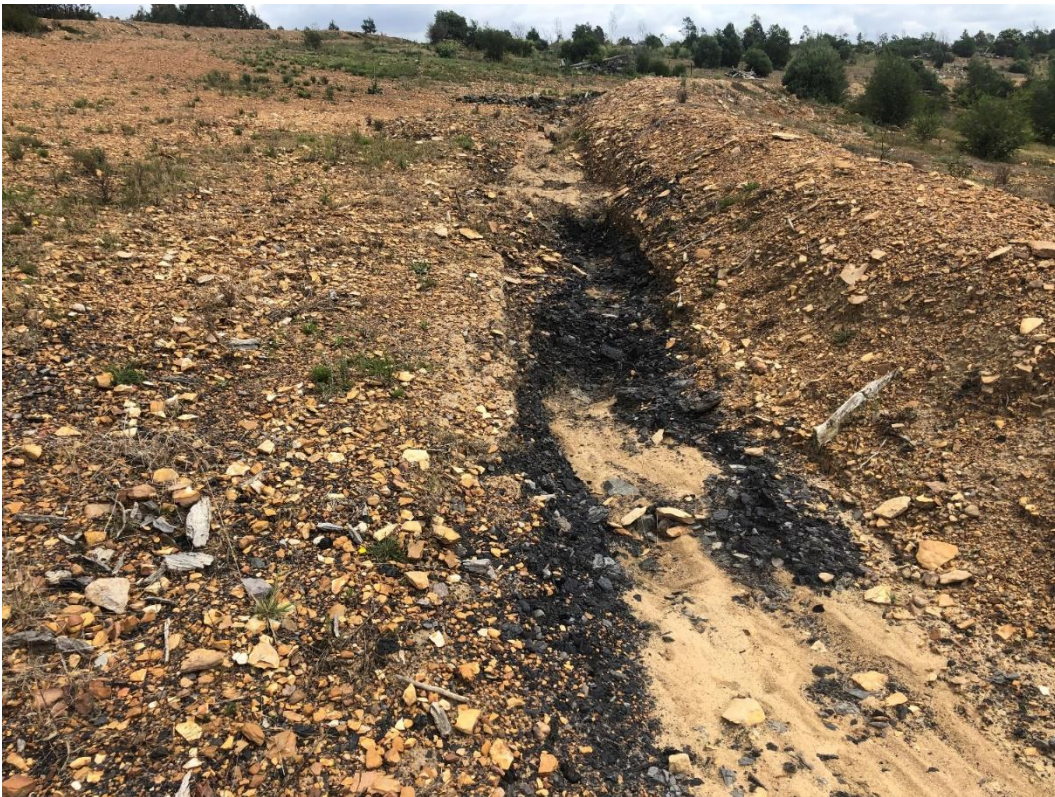
Photo 12 Some evidence of erosion in contour bank without rock armour
