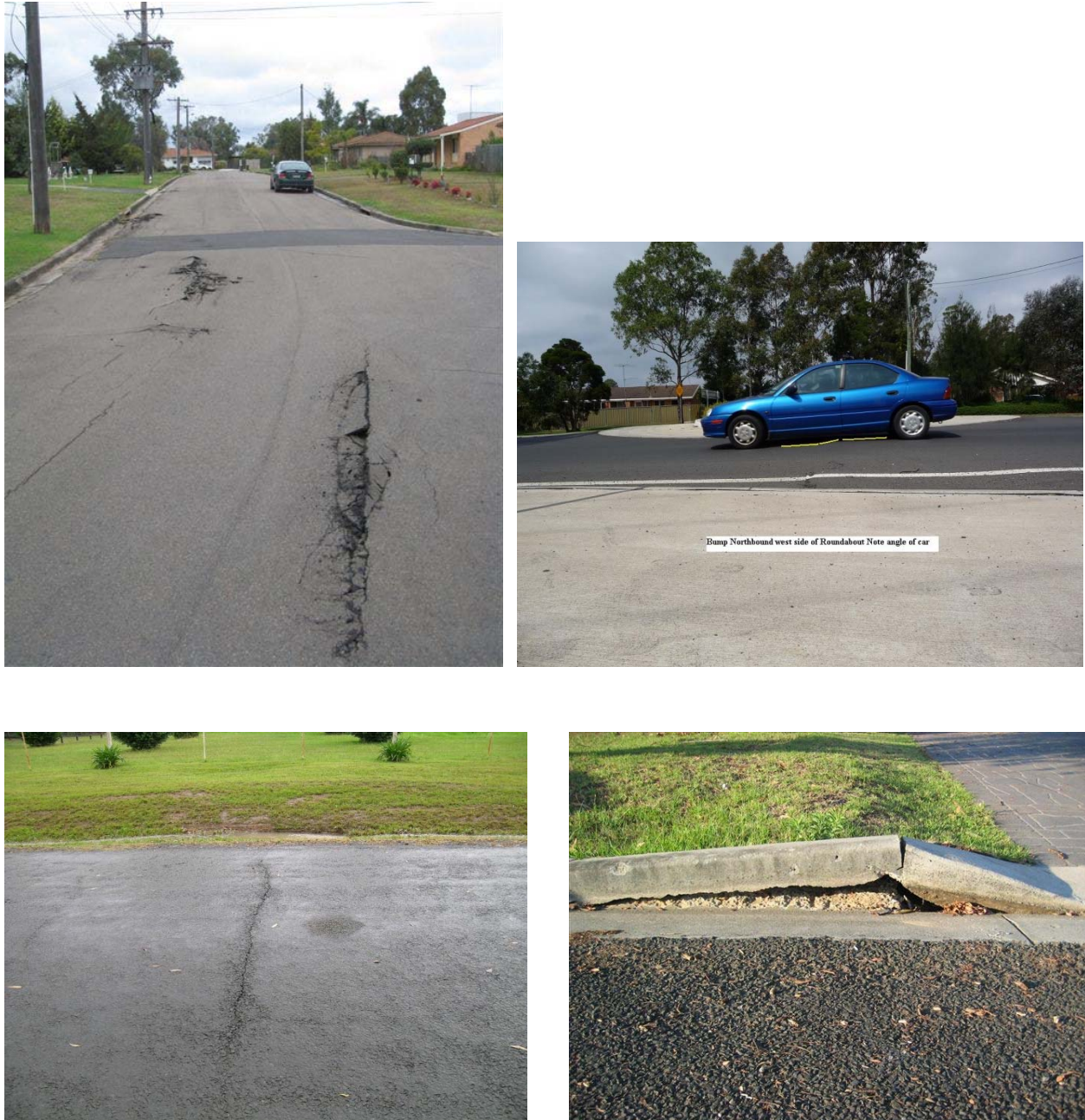
Fig. 6.18 Previously Observed Impacts on Local Roads above Tahmoor Mine
