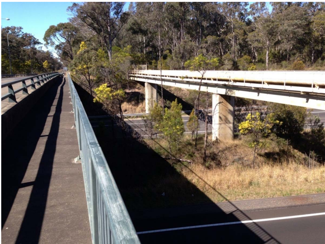
Fig. 6.13 Water Pipe Bridge over M31 Hume Motorway adjacent to Avon Dam Road
