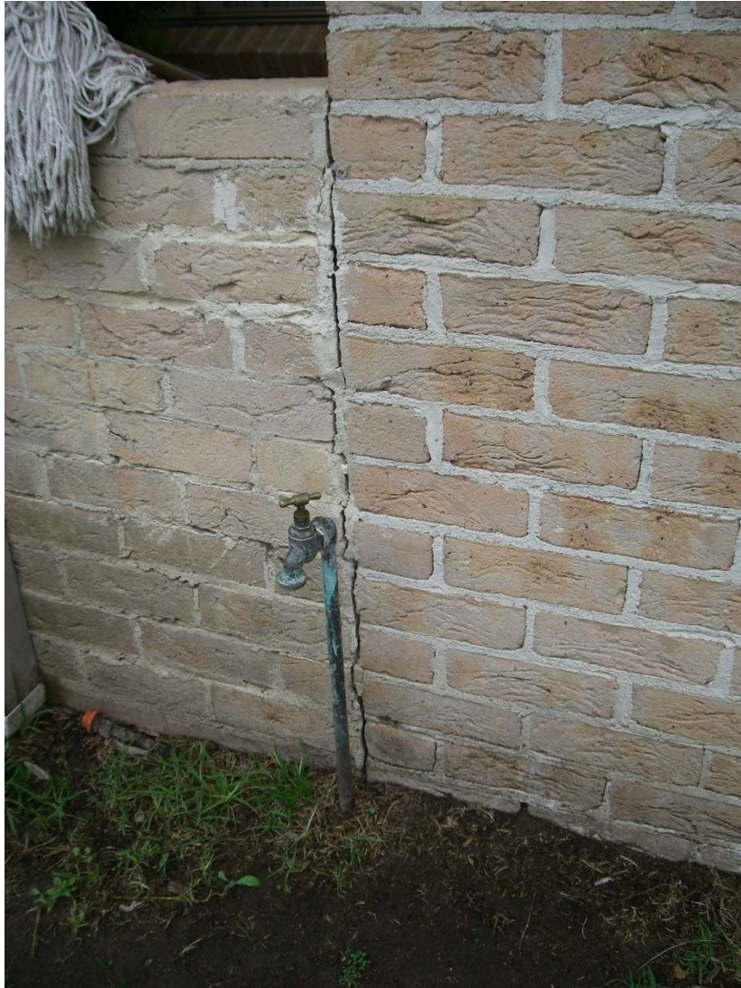
Fig. C.2 Example of crack in mortar only
