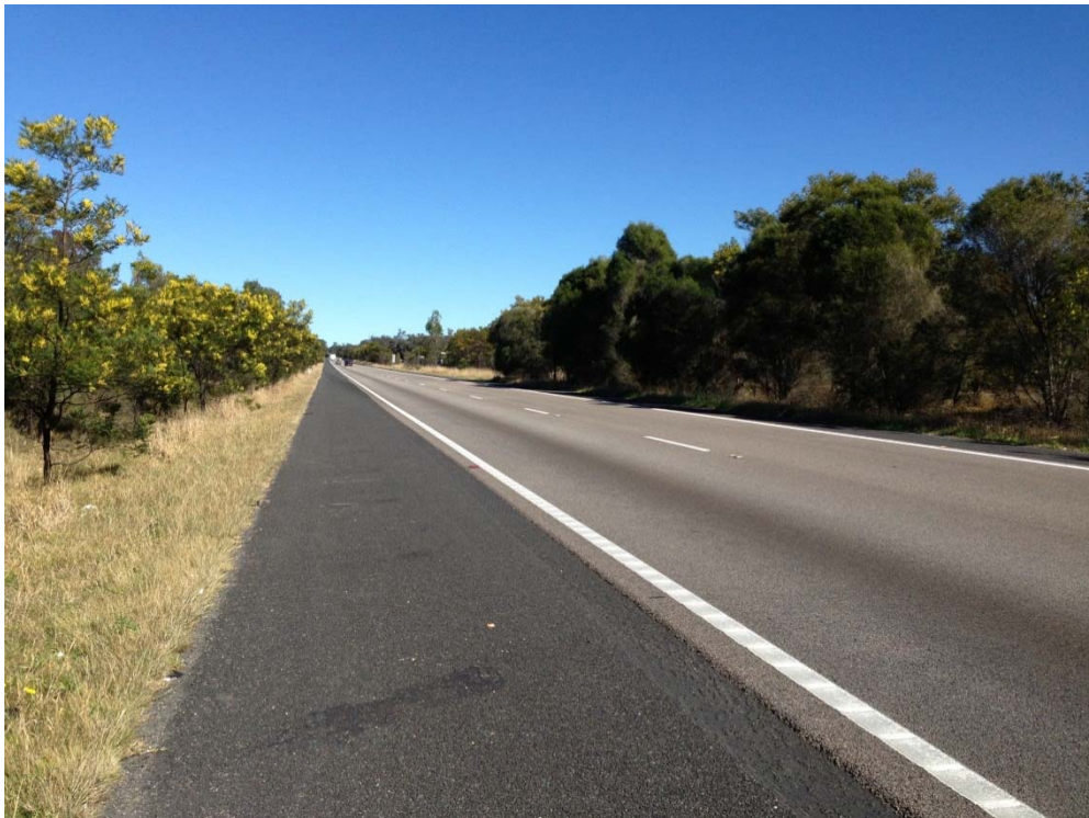
Fig. 6.8 Southbound Carriageway of M31 Hume Motorway near the Subsidence Study Area
