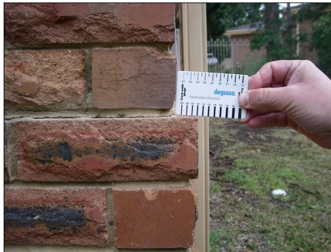
Fig. C.1 Example of slippage on damp proof course
