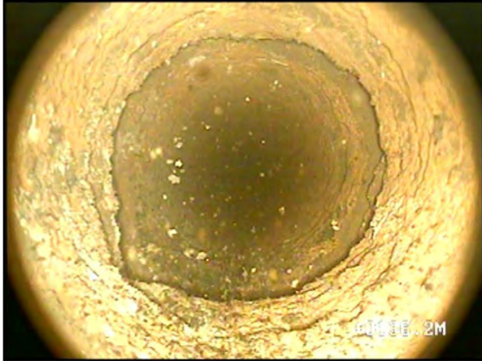
Appendix 6.5: 136.8m - Core loss zone, water loss zone, horizontal joint zone & small cavity.
