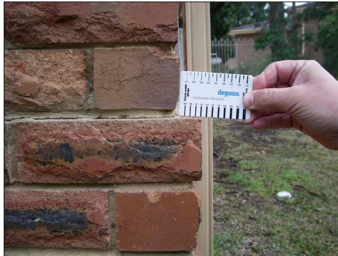
Fig. B.1 Example of slippage on damp proof course
