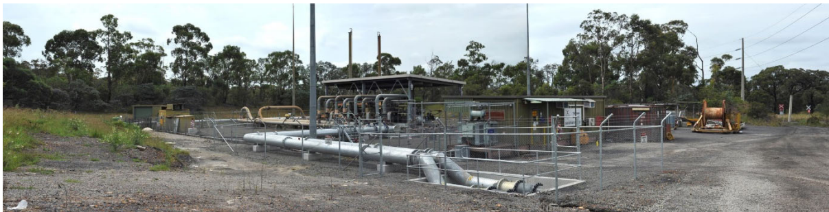
Plate 8 – Existing on-site gas plant within Tahmoor Mine surface facility
