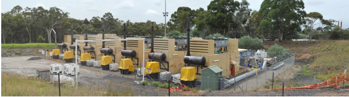
Plate 7 – Existing cogeneration plant within Tahmoor Mine surface facility
