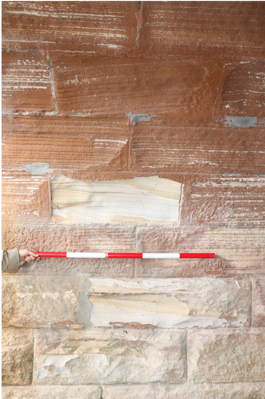
Plate 3.3 Damage to sandstone culvert, chainage 88.980.
