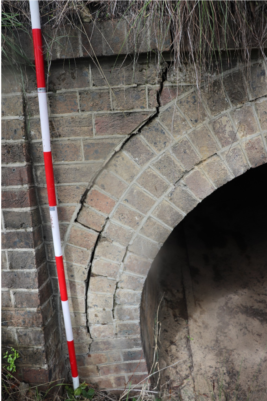
Plate 3.4 Cracking on north entrance to culvert at chainage 87.300. View south.
