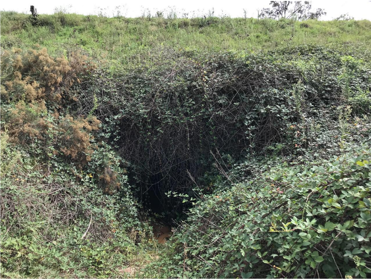
Plate 3.1 Sandstone culvert, chainage 88.400, overgrown with weeds and brambles. View west.
