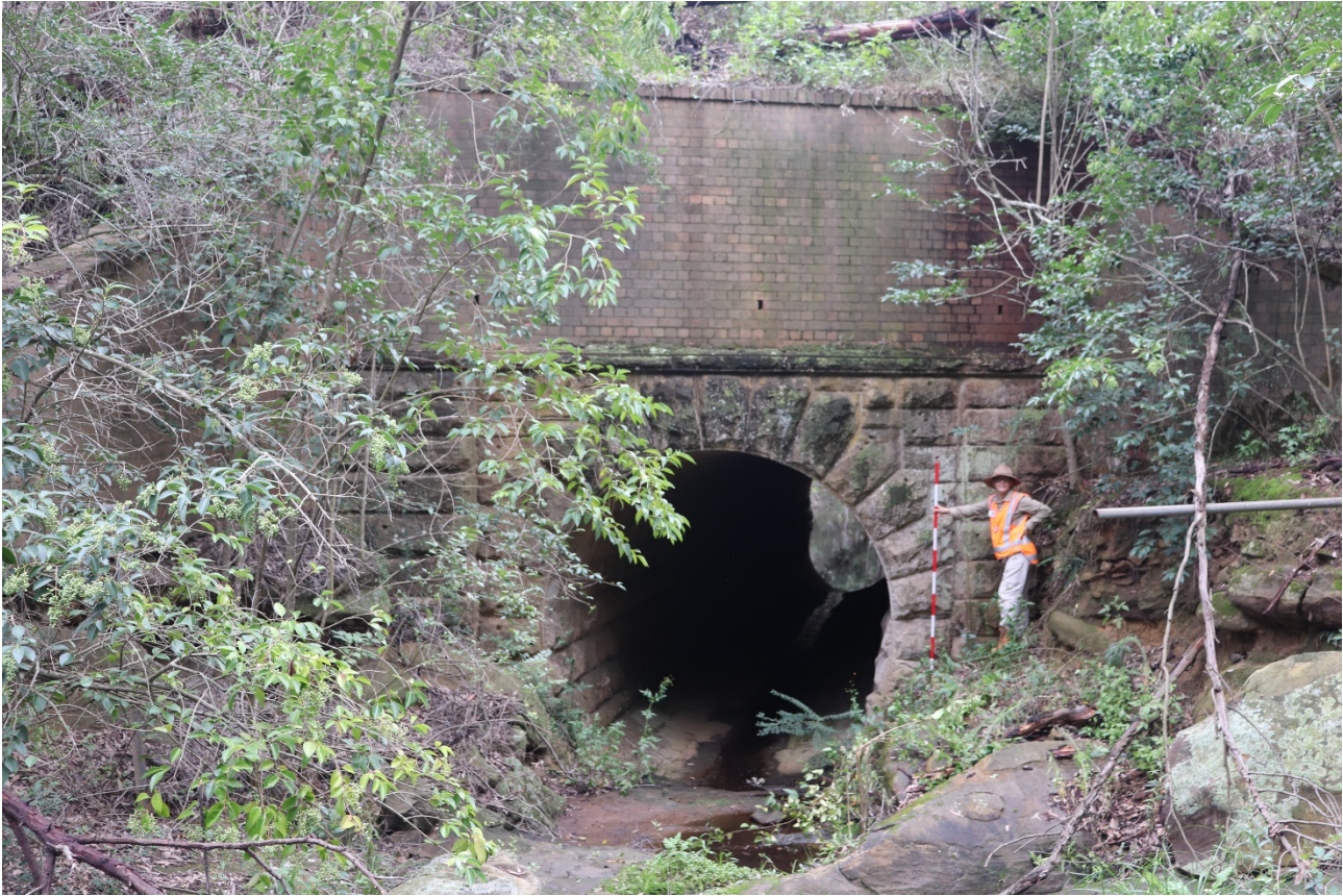
Plate 3.5 Sandstone culvert with the later addition of brick wingwalls and head wall (chainage 89.629). View west.
