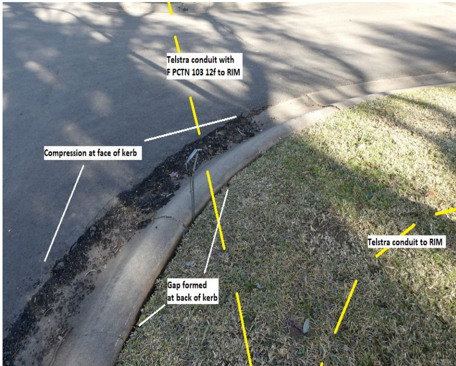
Plate 4: View of compression above Telstra conduit at northern end of Stonequarry Creek Rd adjacent to RIM PCTJ.
