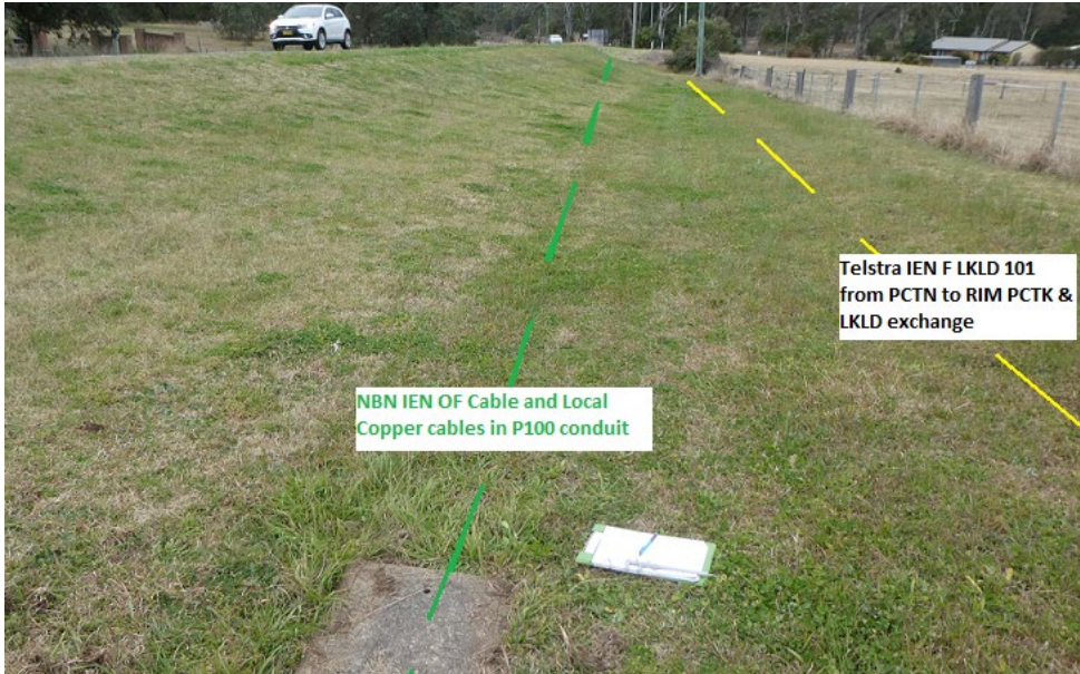
Plate 5: View of No 6 Pit in Barkers Lodge Road looking east towards PCTN Exchange showing alignment of direct buried Telstra optical fibre cable F LKLD 101 18f installed along the southern side of the road alignment within the road reserve adjacent to fence line.
