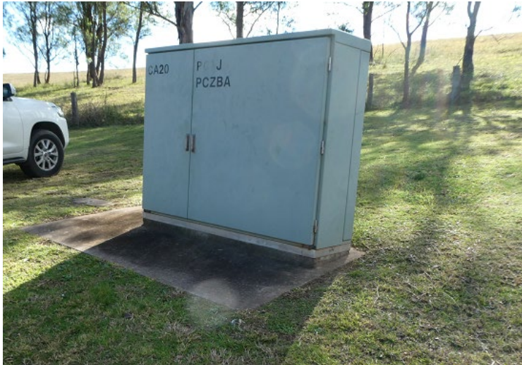
Plate 6: View of RIM PCTJ located at the northern end of Stonequarry Creek Road over the eastern extraction edge of LW W1. This RIM is fed by IEN optical fibre cable F PCTN 103 from Picton exchange with a 12f optical fibre cable spur line along Stonequarry Creek Road from the joint at Thirlmere Way.
