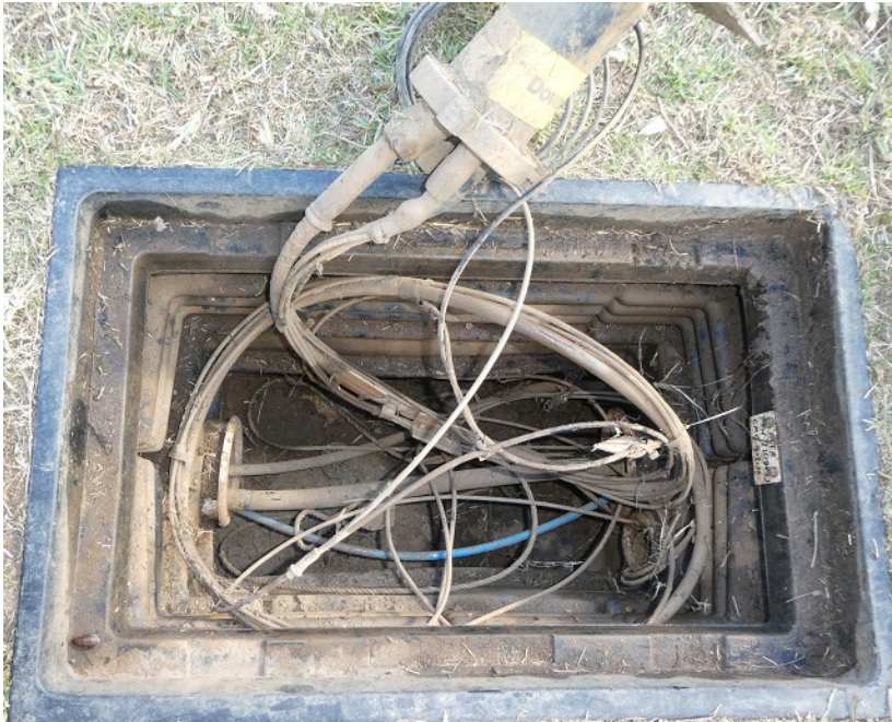
Plate 3: View into typical Telstra plastic pit showing Telstra P100 conduit and pit and NBNSCo Local copper distribution cables along Stonequarry Creek Road. Note blue cable is Telstra optical fibre cable
