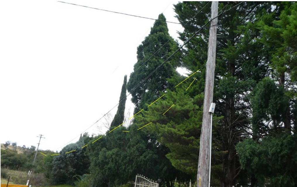
Plate 6: View of NBNC Co Local aerial cable west at western end of Connellan Crescent near the intersection with Rumker St.
