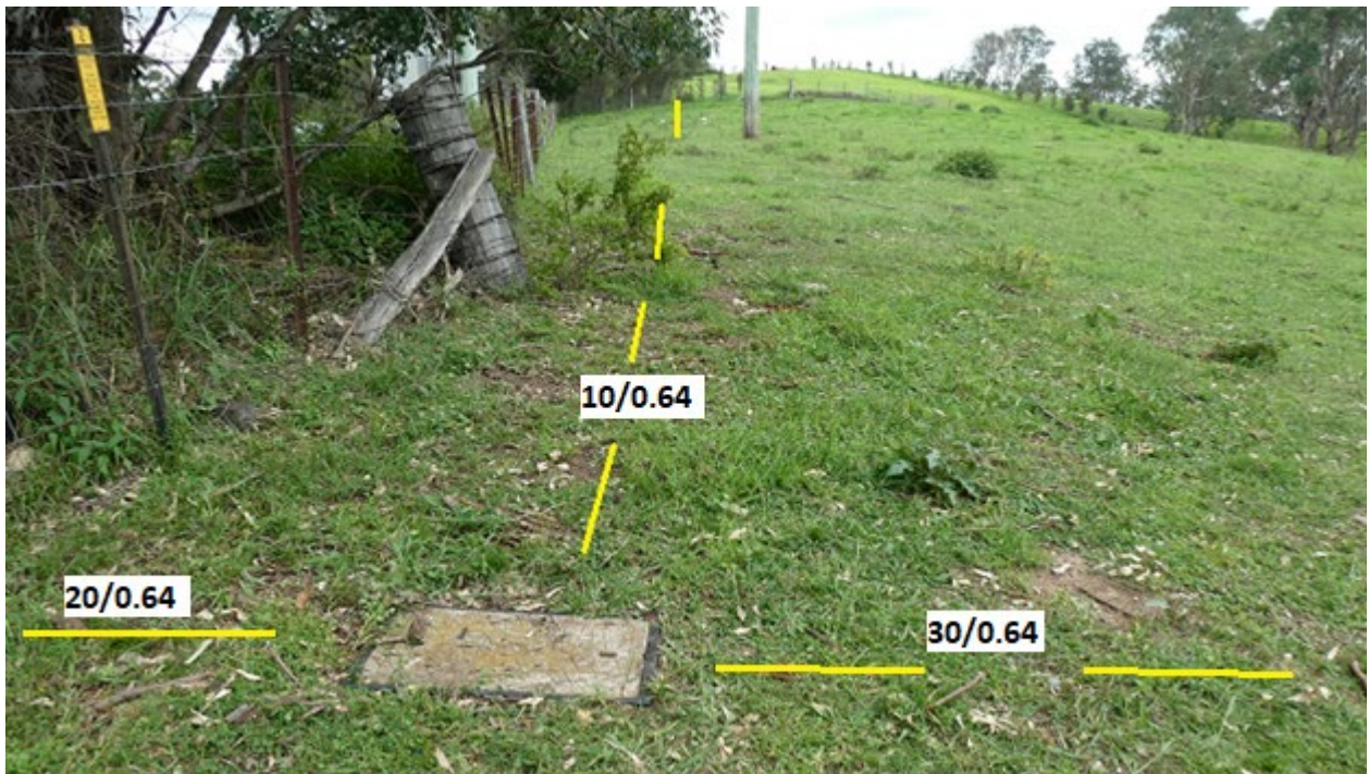
Plate 4: View of Telstra No5 Pit in private property on north side of Thirlmere Way outside the Study Area. Photo shows line of NBNSCo cable 30/0.64 from across LW W3 W4 inside Study Area, north-west 10/0.64 to two properties outside the Study Area and 20/0.64 crossing Thirlmere Way to the south outside the Study Area. See Plate 1 showing crossing Thirlmere Way outside the Study Area. Cables are grease filled hard jacket resilient cables.
