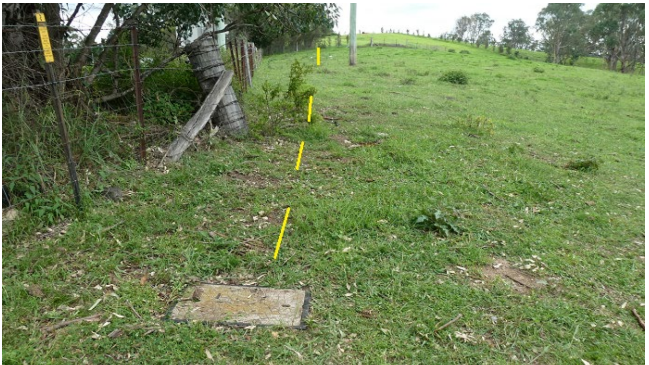
Plate 2.1 View of Telstra No5 Pit in private property on north side of Thirlmere Way showing line of NBNCable cable towards the south east corner of LW W1. Cable is grease filled hard jacket 10/0.64 cable
