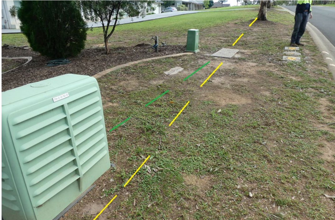
Plate 5 View of NBNC Co Node '2TAH02-07-FNO-001' located at No 13 Stonequarry Creek Road showing NBNC Co (green) and Telstra (yellow) conduit from Telstra No6 Pit to Node and along western side of Stonequarry Creek Road. Note NBNC Co Nodes are not located over LW W1
