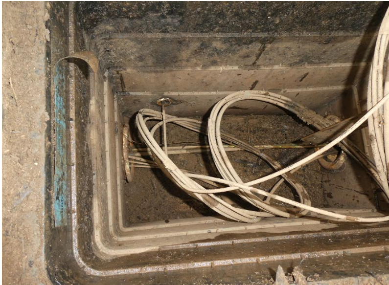
Plate 2.1 View into typical Telstra plastic pit showing P100 conduit and NBNCable cables along Stonequarry Creek Road.
