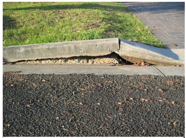
Patterson Street (typical impact to kerb)
