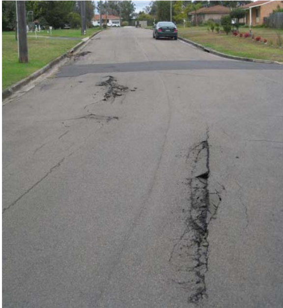
Lintina Street (most severe to date)
