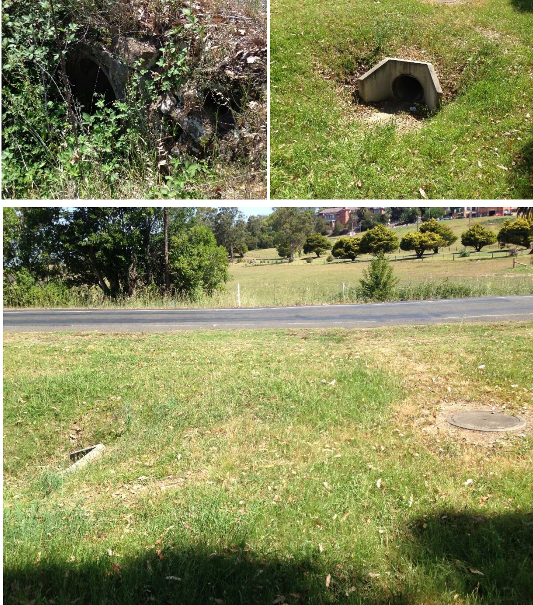
Fig. 3.12 Culvert TH-C2 on Thirlmere Way west of LW W1 with inlet at top left, side inlet in top right and access cover to main culvert in bottom right
