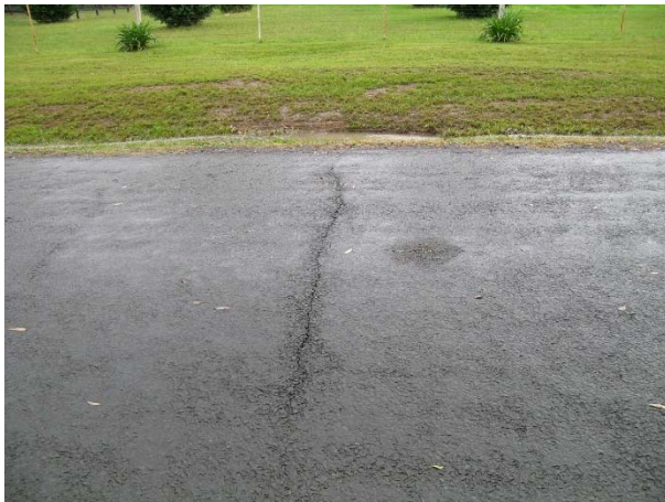
Brundah Road (typical impact to pavement)
