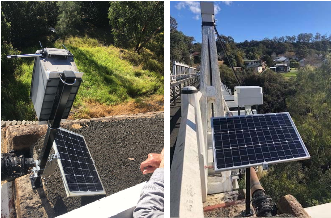
Fig. 2.45 Damaged old and new GNSS Unit 3 at Victoria Bridge on Eastern Abutment B
