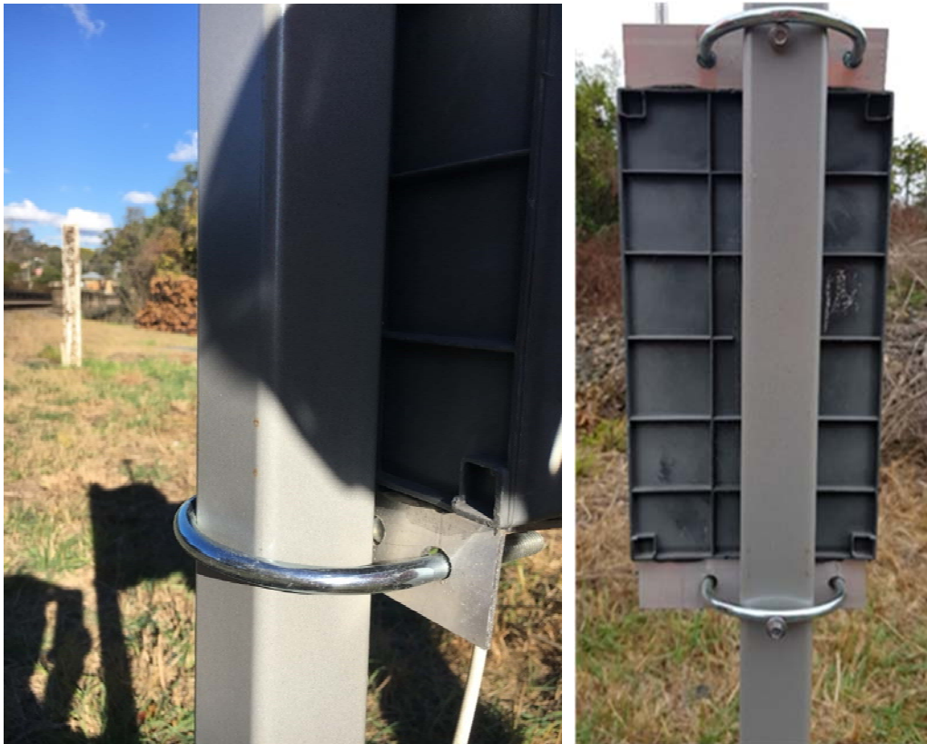
Fig. 2.33 Observed slippage of U-bolt down the post at northern GNSS unit
