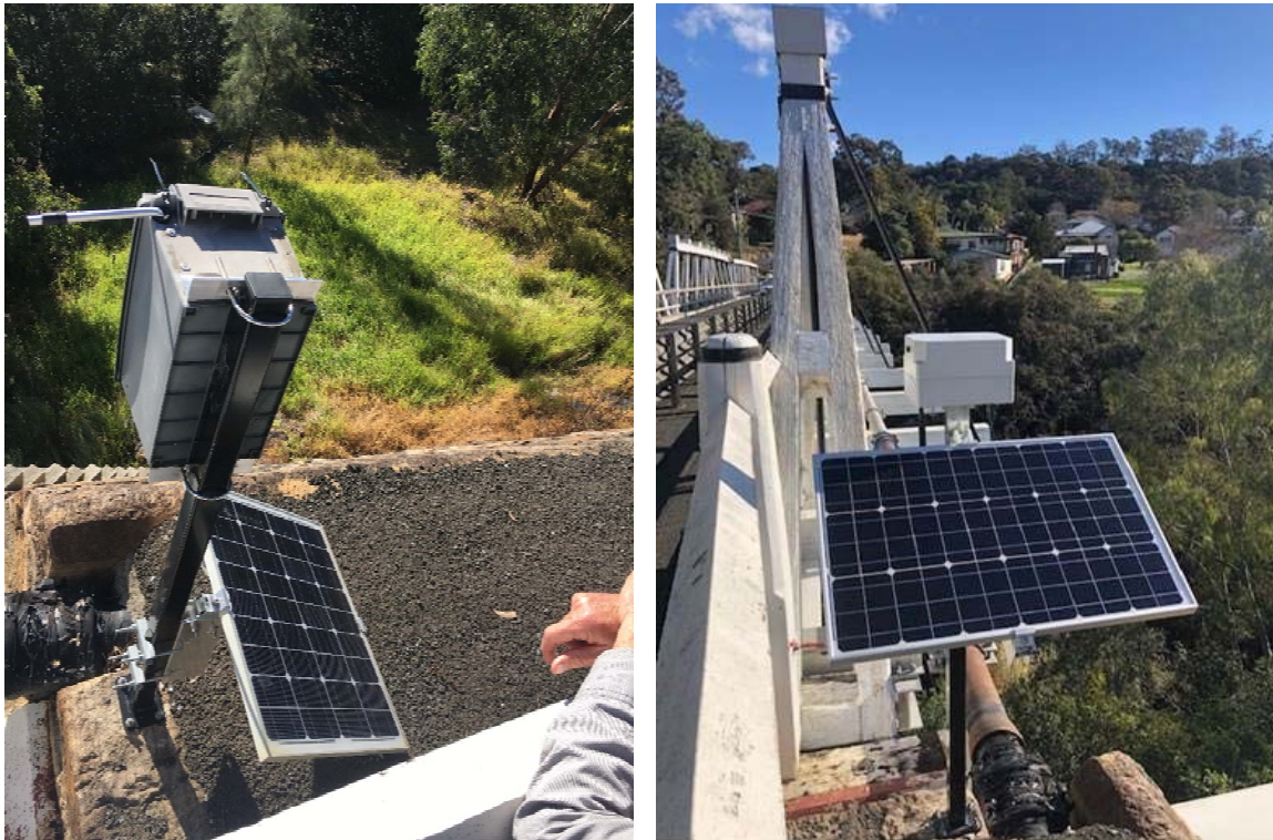
Fig. 2.40 Damaged old and new GNSS Unit 3 at Victoria Bridge on Eastern Abutment B
