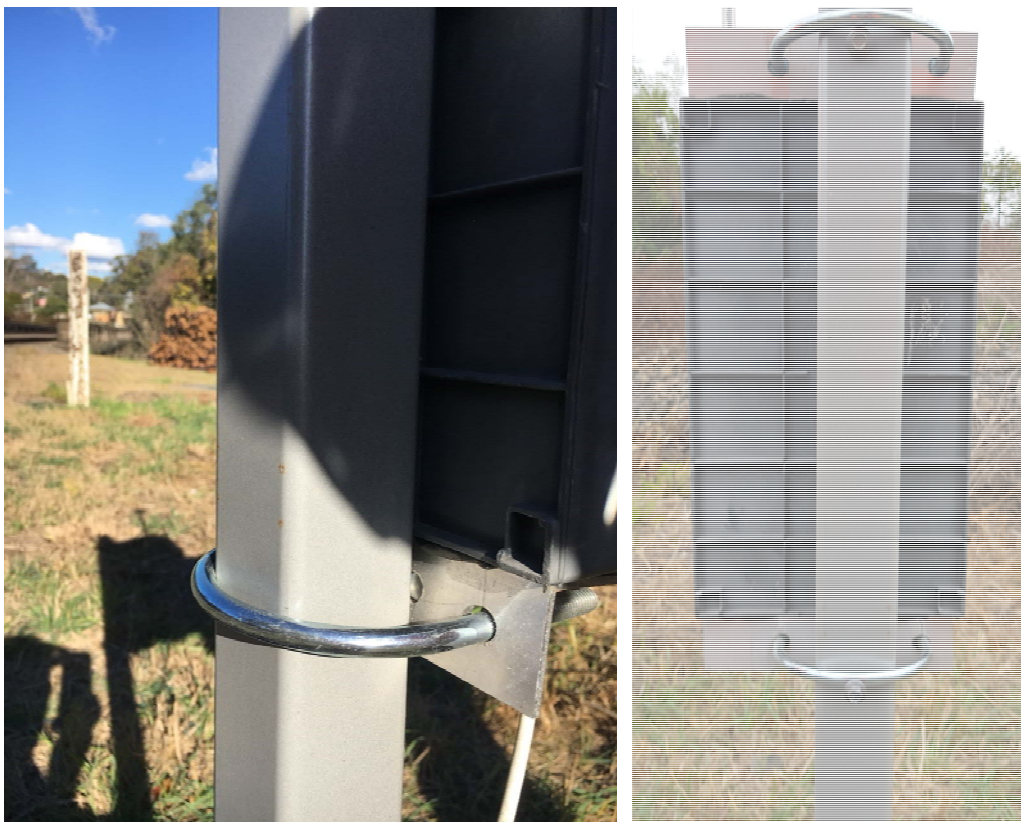
Fig. 2.30 Observed slippage of U-bolt down the post at northern GNSS unit
