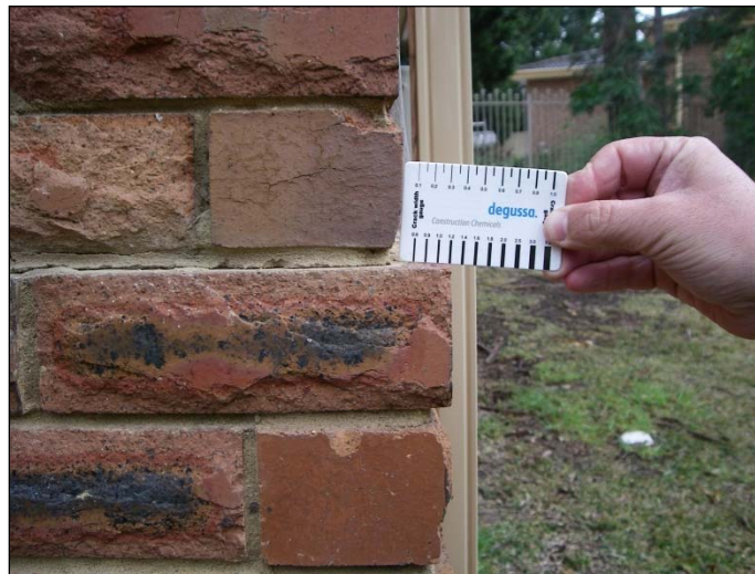
Fig. C.1 Example of slippage on damp proof course
