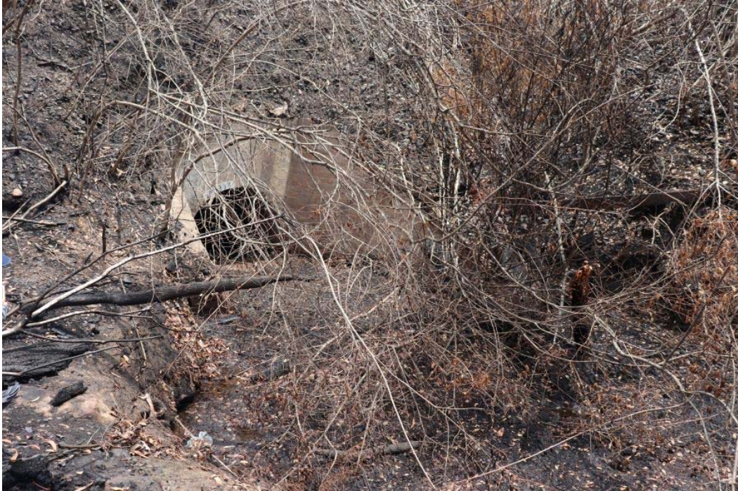
Plate A.10 Culvert 99.338 on Tea Tree Creek under the rail line. View north-west.
