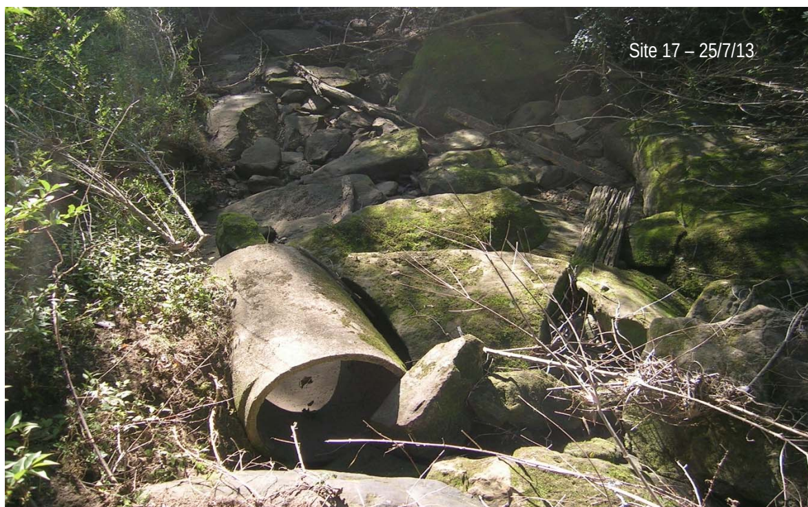
Figure 10 Site 11 and 17 Subsidence Effects after Longwall 27 Extraction
