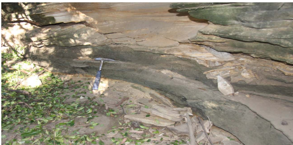
Figure 3 Cracking over Longwall 25
