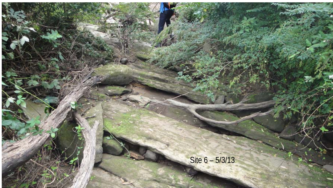
Figure 4 Site 5 and 6 Subsidence Effects after Longwall 26 Extraction
