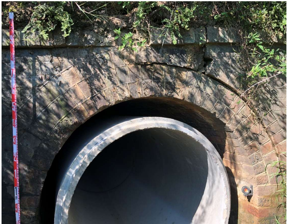
Cracking and displacement of bricks around the western portal arch. Does not appear to have worsened during longwall mining in the Western Domain.
