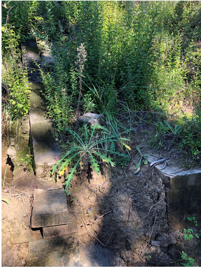
Displaced bricks at the base of the brick chute to the south of the eastern portal.
