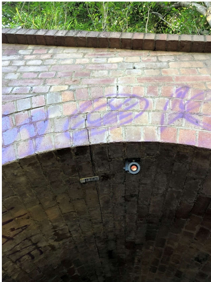
Western portal. Cracking through the mortar above the arch continues along the roof of the culvert.
