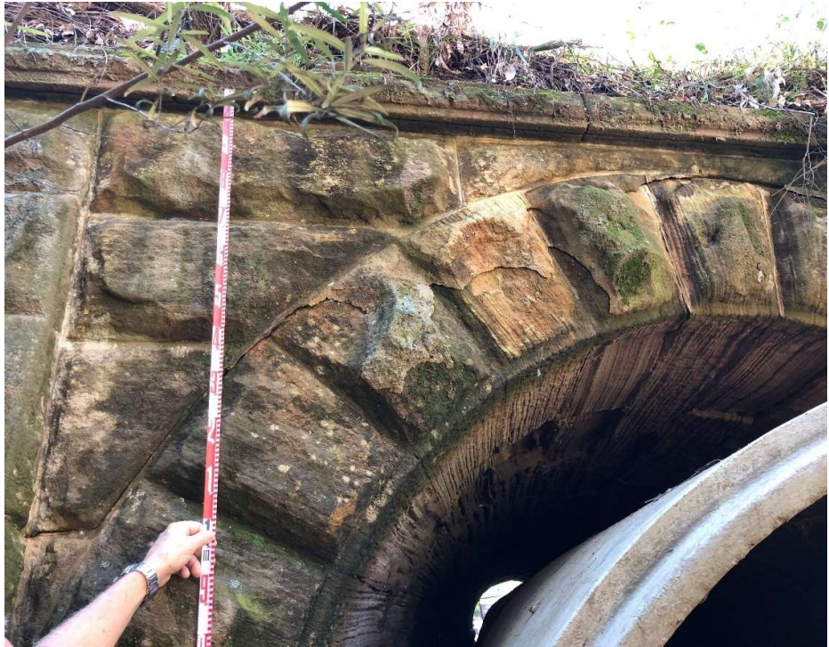
Western portal. Cracking along the mortar and spalling of the arch stones has not worsened significantly during extraction of LW W3.
