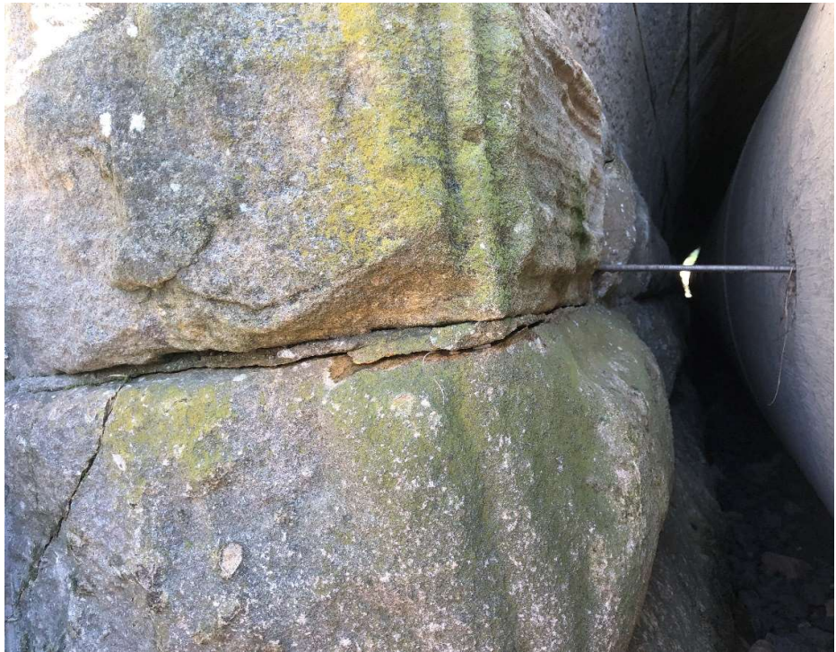
Eastern portal. Screw securing concrete sleeve to the arch of the culvert has resulted in some cracking along the mortar and through the sandstone.
