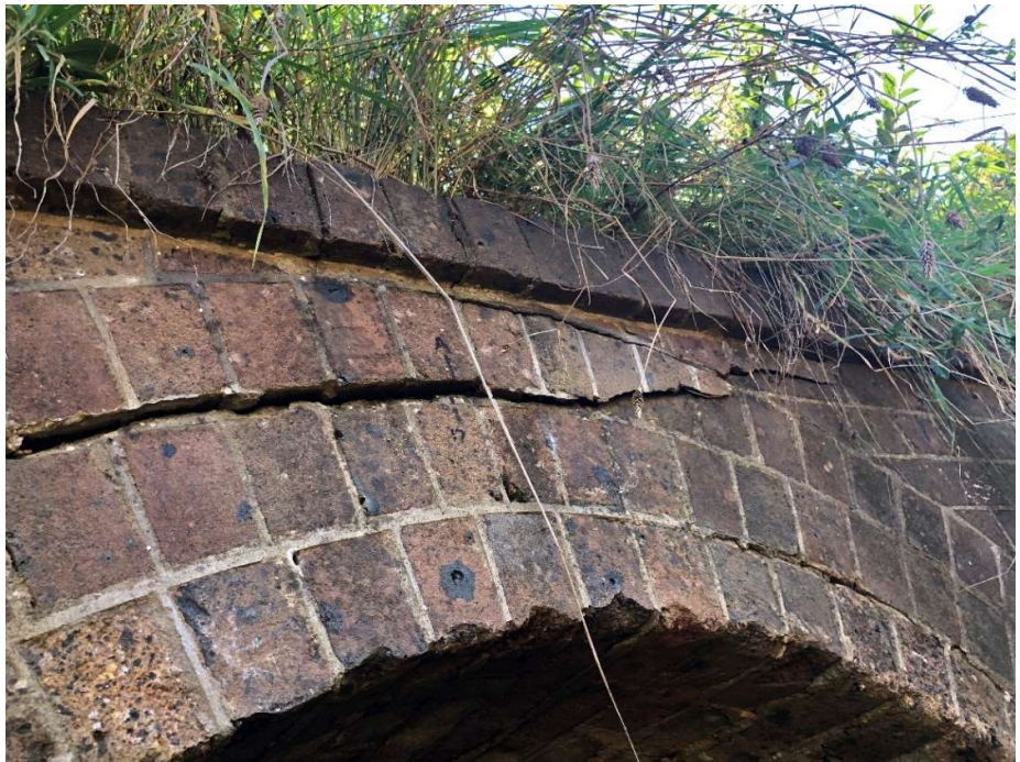
Detail, pre-existing cracking and displacement of bricks around the eastern portal arch that does not appear to have worsened significantly during longwall mining in the Western Domain.
