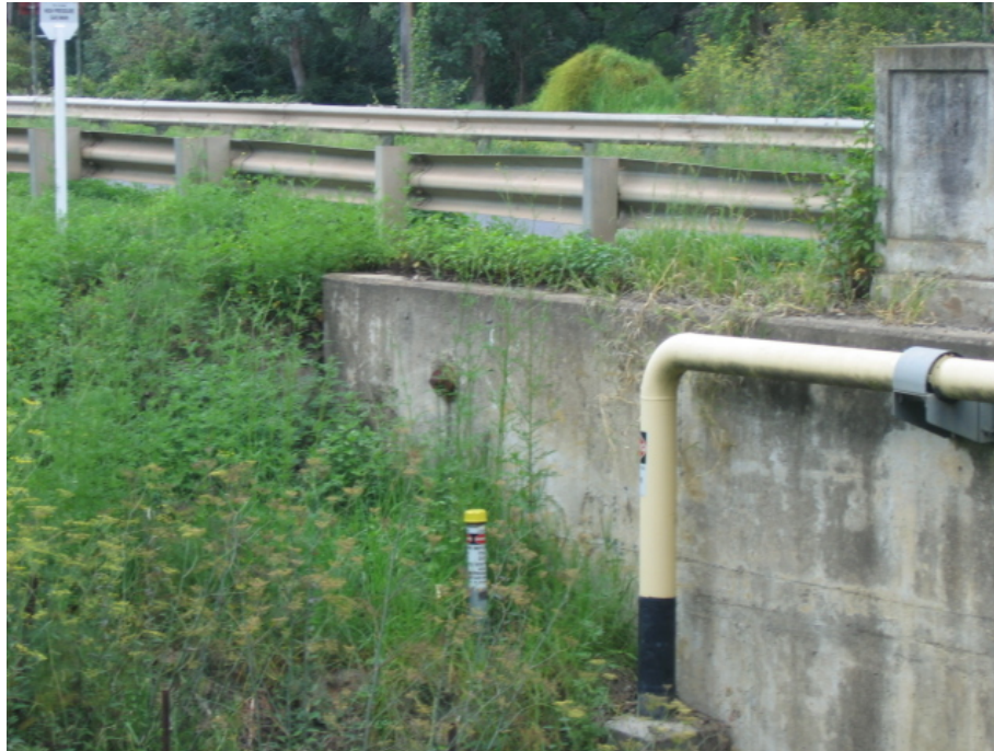
Fig. 3.13 Termination of steel gas pipe at end of Remembrance Drive Road Bridge
