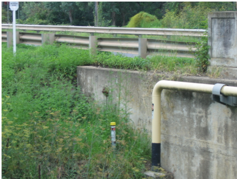
Fig. 3.16 Termination of steel gas pipe at end of Remembrance Drive Road Bridge
