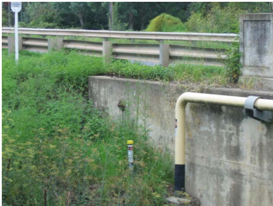
Fig. 3.9 Termination of steel gas pipe at end of Remembrance Drive Road Bridge
