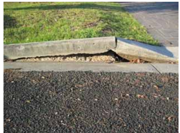
Patterson Street (typical impact to kerb)
