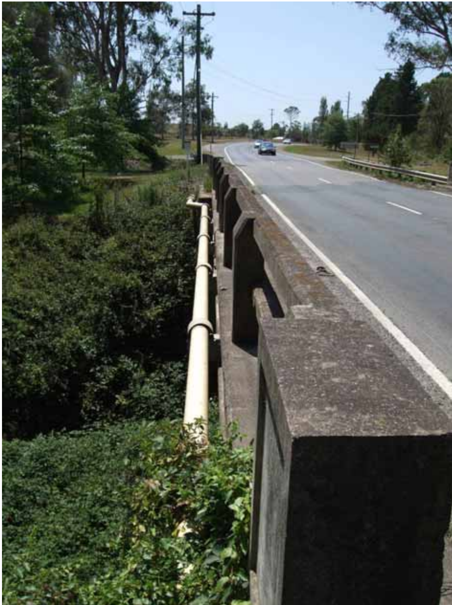
Figure 11 Gas pipe support along bridge.
