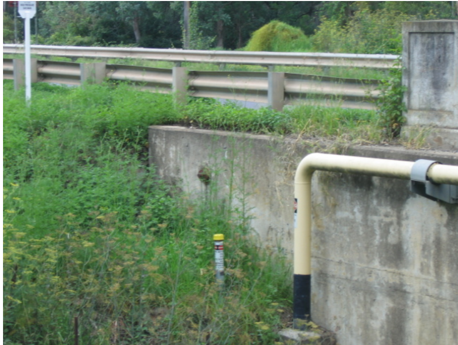
Fig. 3.11 Termination of steel gas pipe at end of Remembrance Drive Road Bridge
