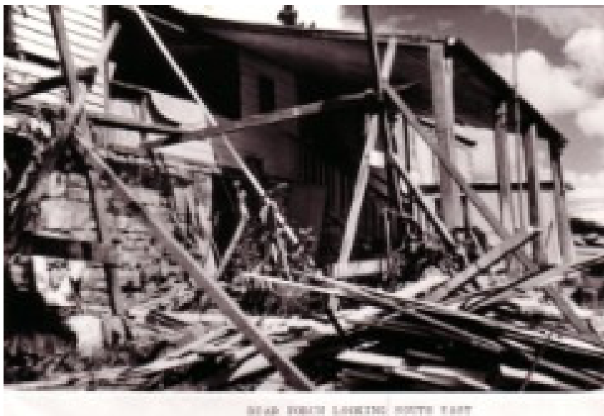
Figure 47 Dilapidated structure adjacent to northwestern corner of the dwelling circa 1972
