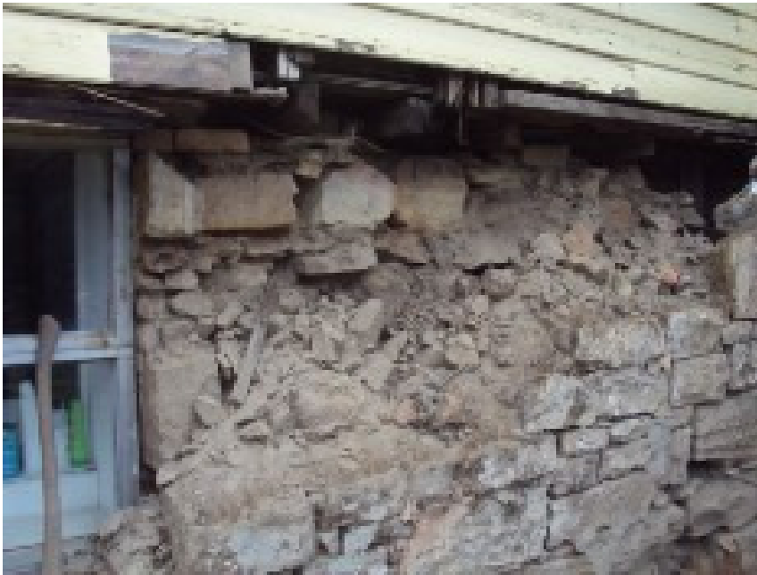
Figure 50 Mortar erosion exposed when the external brickwork was removed near the northwest corner of the dwelling during recent renovation.
