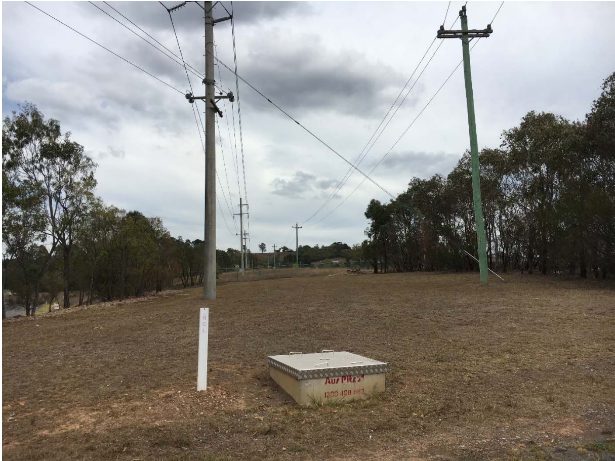
Fig. 3.14 66kV Powerline (left) and 11kV Powerline (right) within Sydney Water's Picton Water Recycling Plant
