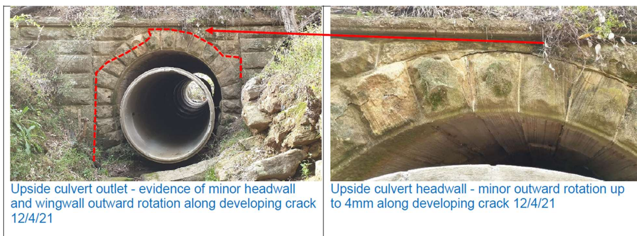
Figure 2-3 Cracking at culvert 88.980 km (source: PMLL Detailed Monitoring Report 19, Appendix E ).
