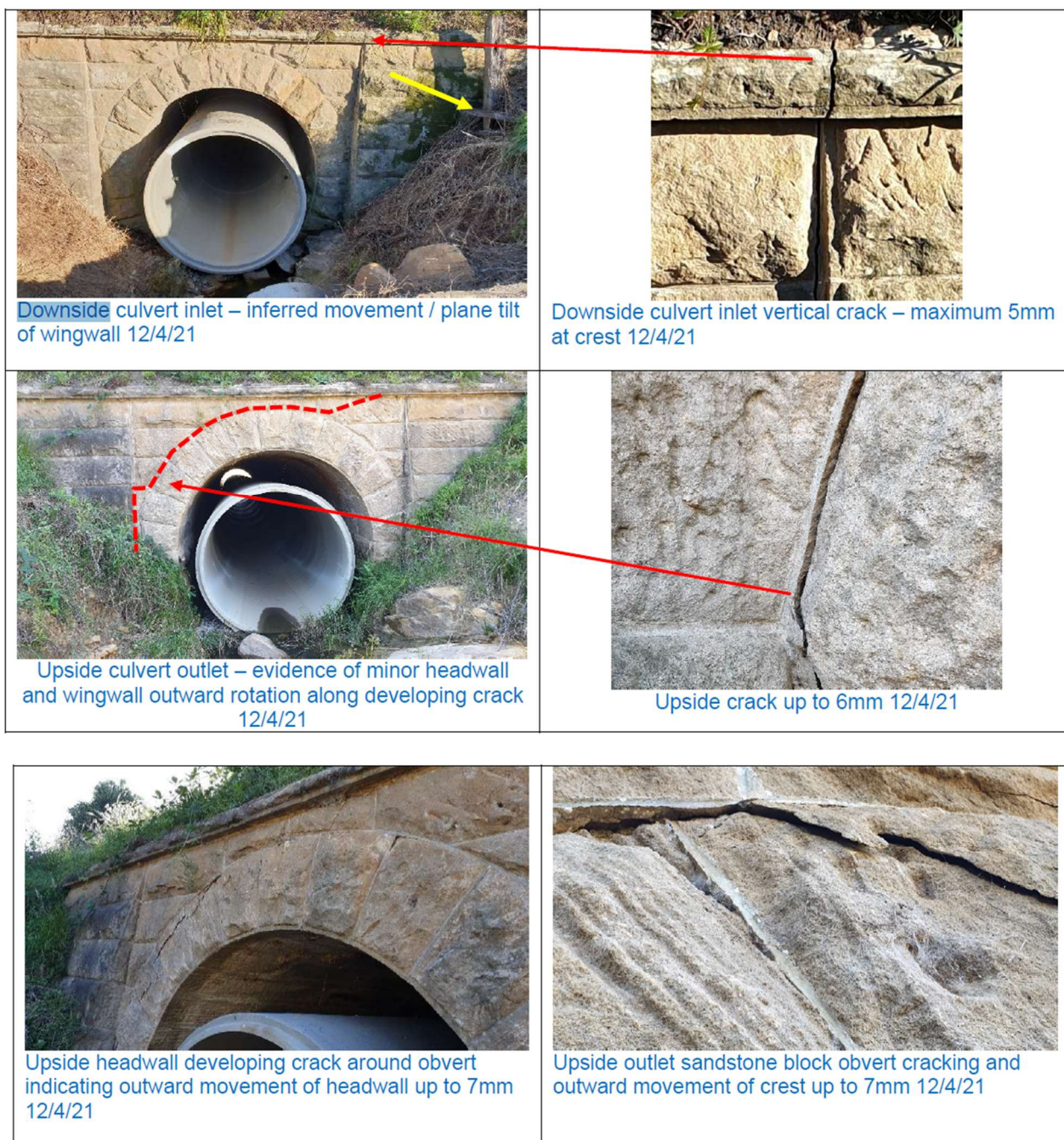
Figure 2-2 Cracking at culvert 88.44 km (source: PMLL Detailed Monitoring Report 19, Appendix E ).
