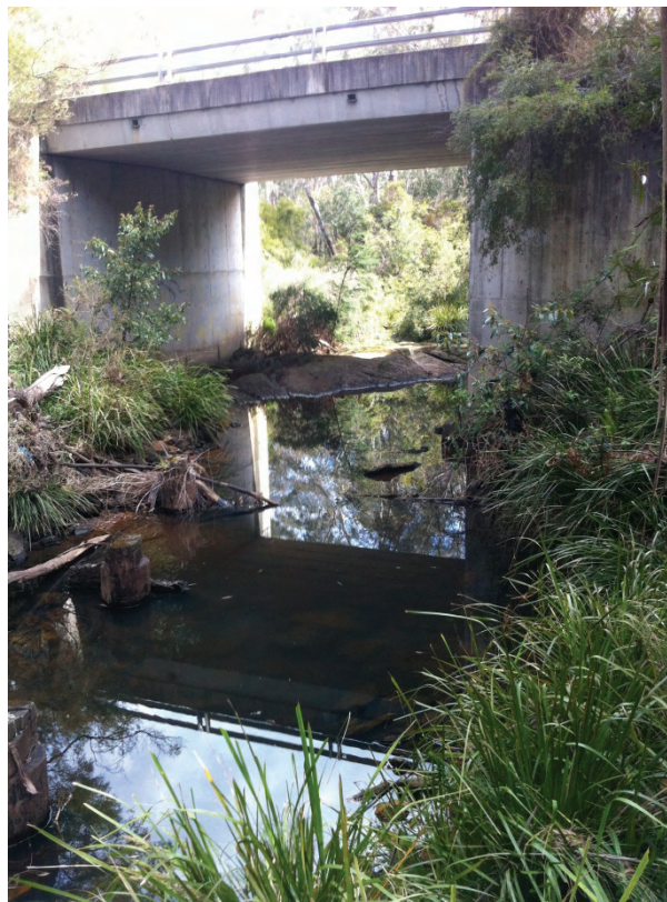
Fig. 5.16 Ponded water in Dog Trap Creek near Bridge over Arina Road above previously extracted Longwall 13, ten years after mining
