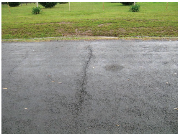
Brundah Road (typical impact to pavement)
