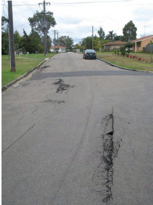
Lintina Street (most severe to date)
