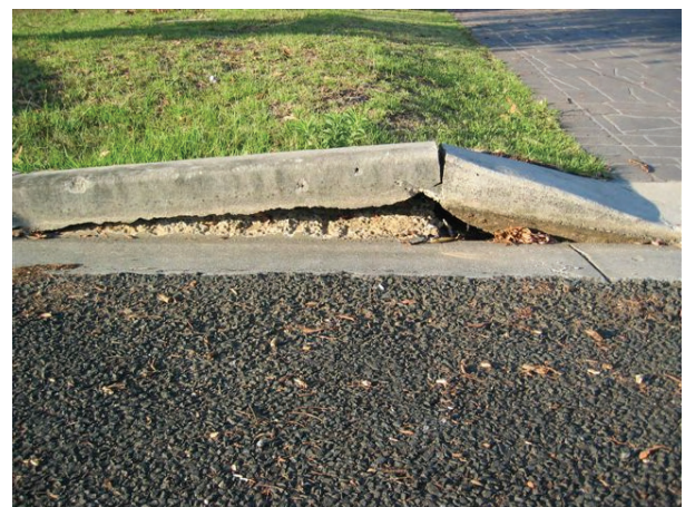
Patterson Street (typical impact to kerb)
