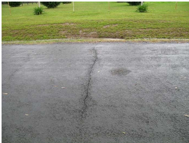
Brundah Road (typical impact to pavement)
