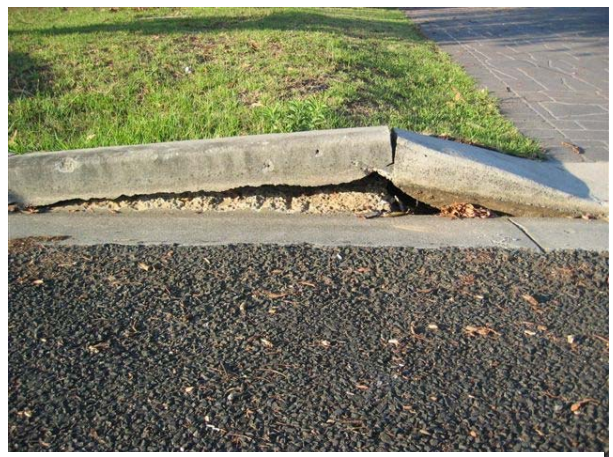
Patterson Street (typical impact to kerb)
