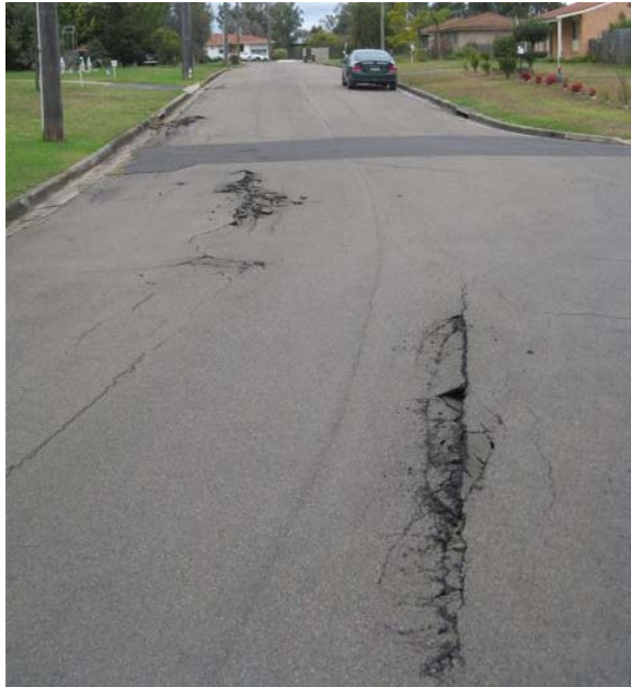
Lintina Street (most severe to date)
