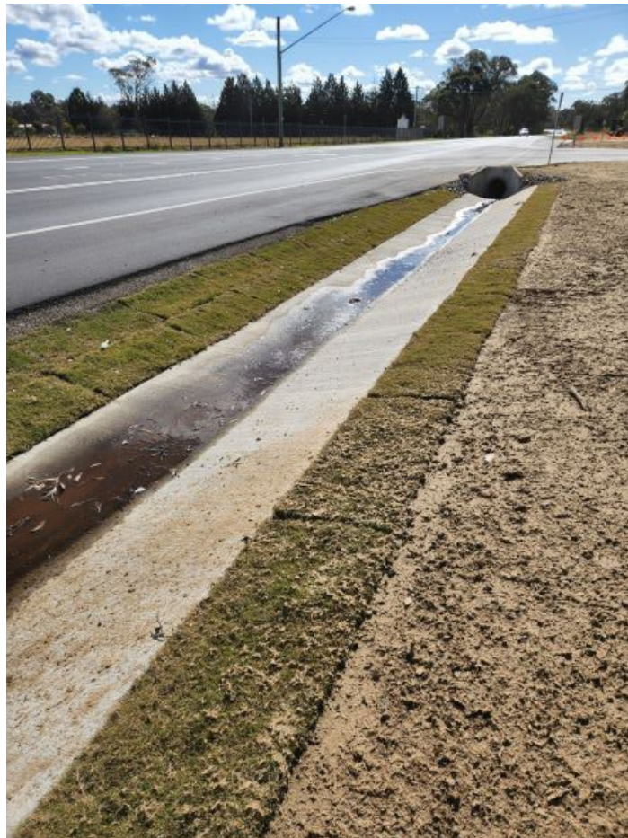
Photo 4 - Concrete and turf lined drain with temporary stabilisation applied to exposed areas
