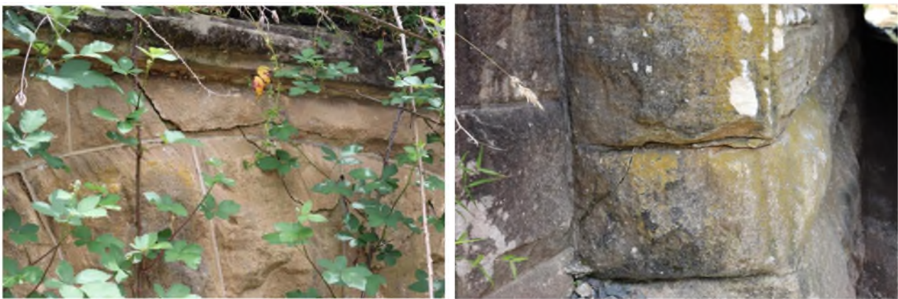
Figure 2-1 Cracking on the portal ends at culvert 88.400 km. This cracking has not worsened during the mining of LW W4.
