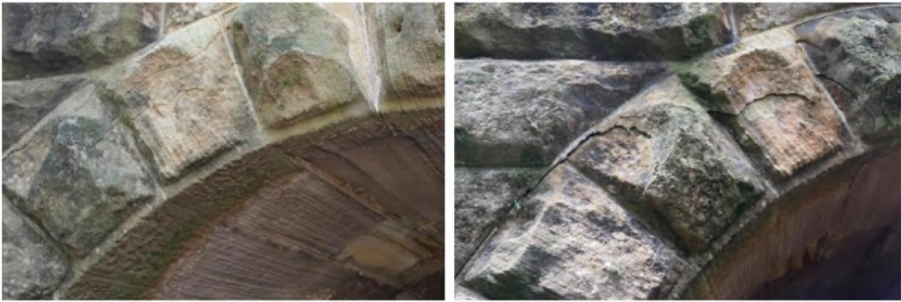
Figure 2-3 Cracking at culvert 88.980 km. Pre-mining (left) and post-mining (right) inspection photographs. Cracking along the mortar and spalling of the arch stones has not worsened significantly during extraction of LW W4.
