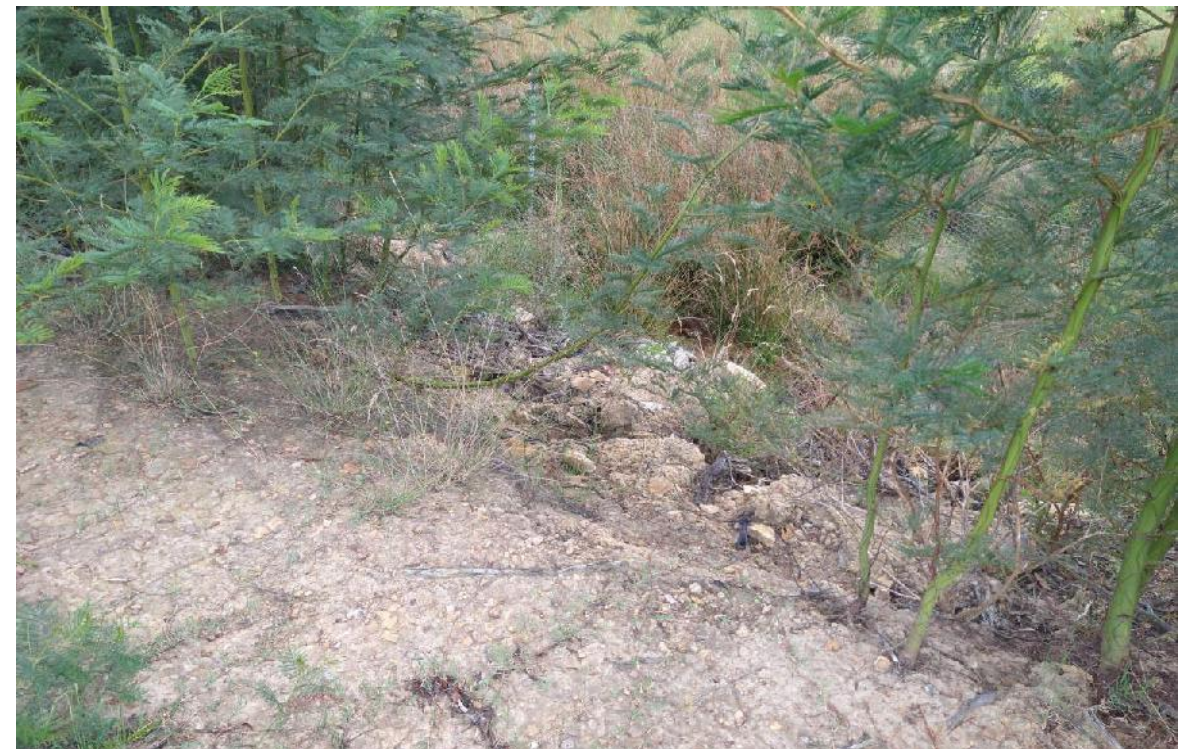
Photo 40: View looking at erosion in the downstream embankment face of FD31. Note: the saplings growing in the downstream face.
