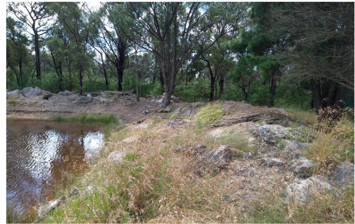
Photo 32: View looking north along the crest and upstream embankment face for FD8. Note: the large sandstone boulders placed over the crest.
