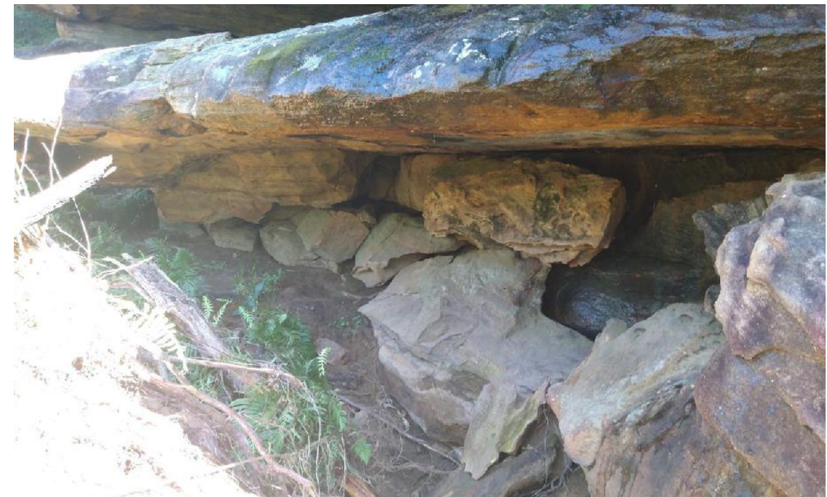
Photo 20: View looking at collapsed joint blocks below a section of overhang near Dekenden Pool (WC2).
