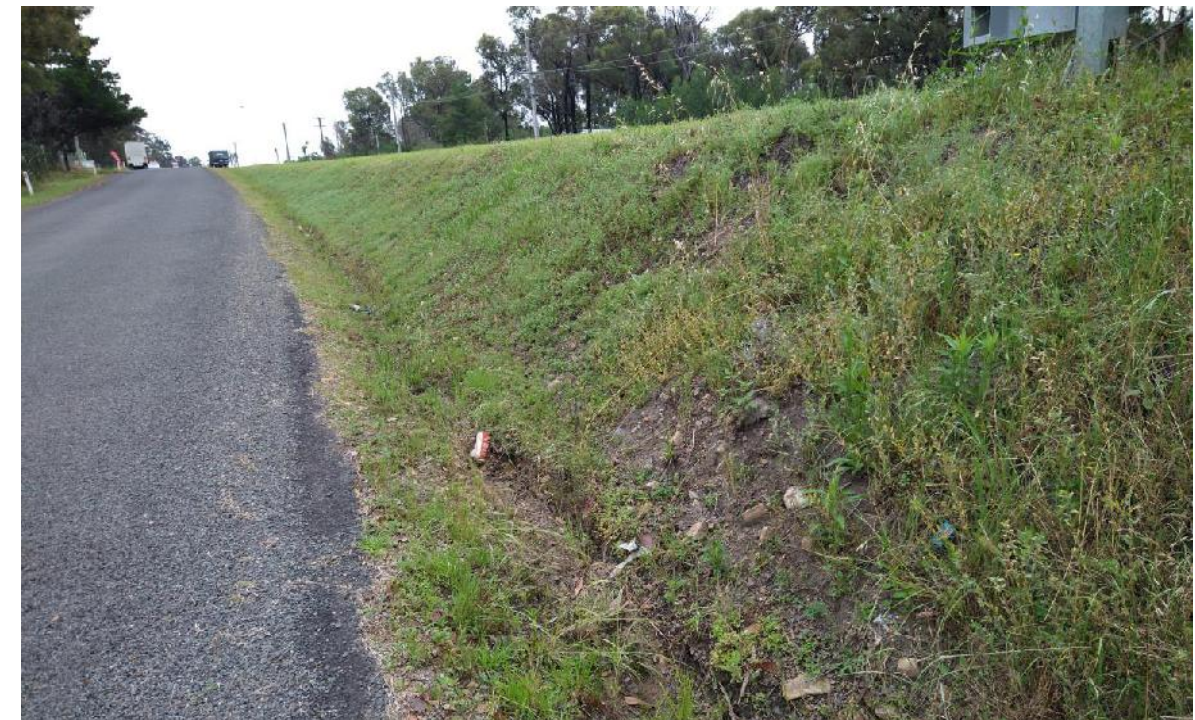
Photo 12: View looking north along the upstream face of RE4 opposite No. 3088 Remembrance Drive.
