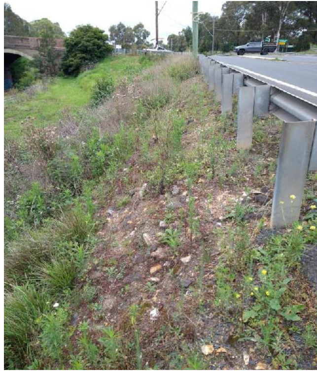
Photo 1: View looking south towards the Wellers Road overpass bridge, along the crest of the downstream face for the RE1 road embankment.
