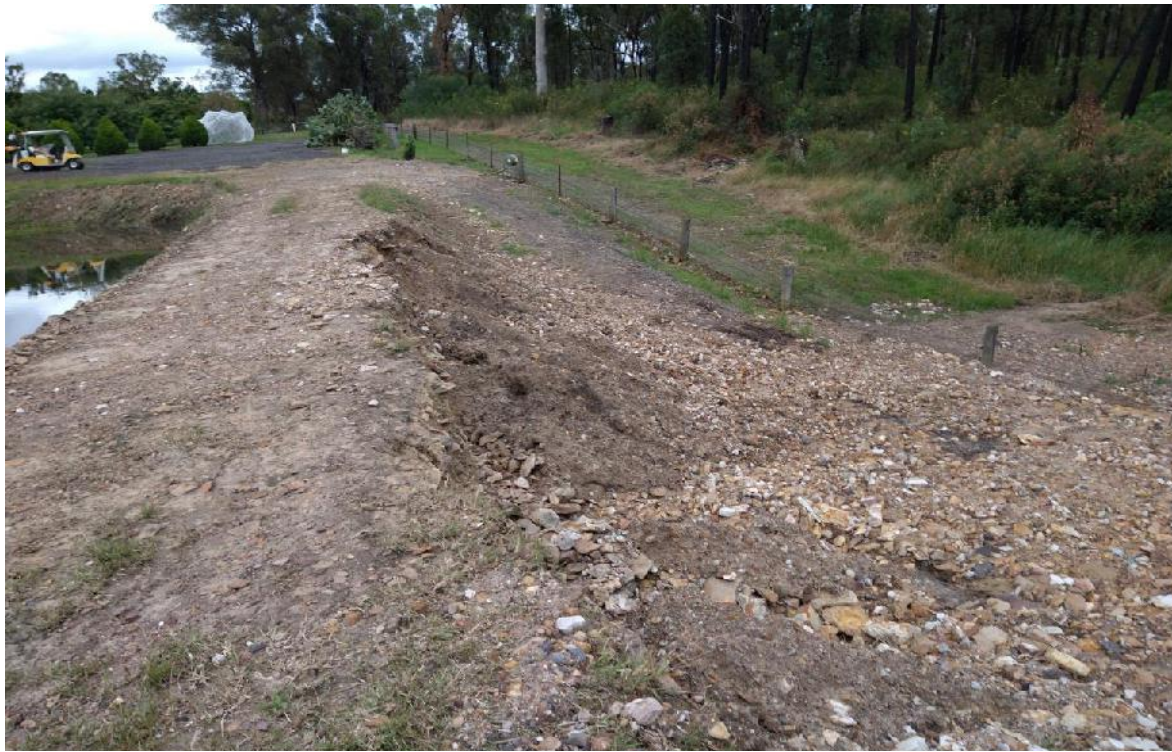
Photo 25: View looking west along the crest of the farm dam at 4 Olive Lane (ie outside SA). Note: the erosion and scour following overtopping during a heavy rainfall event in early April 2022.
