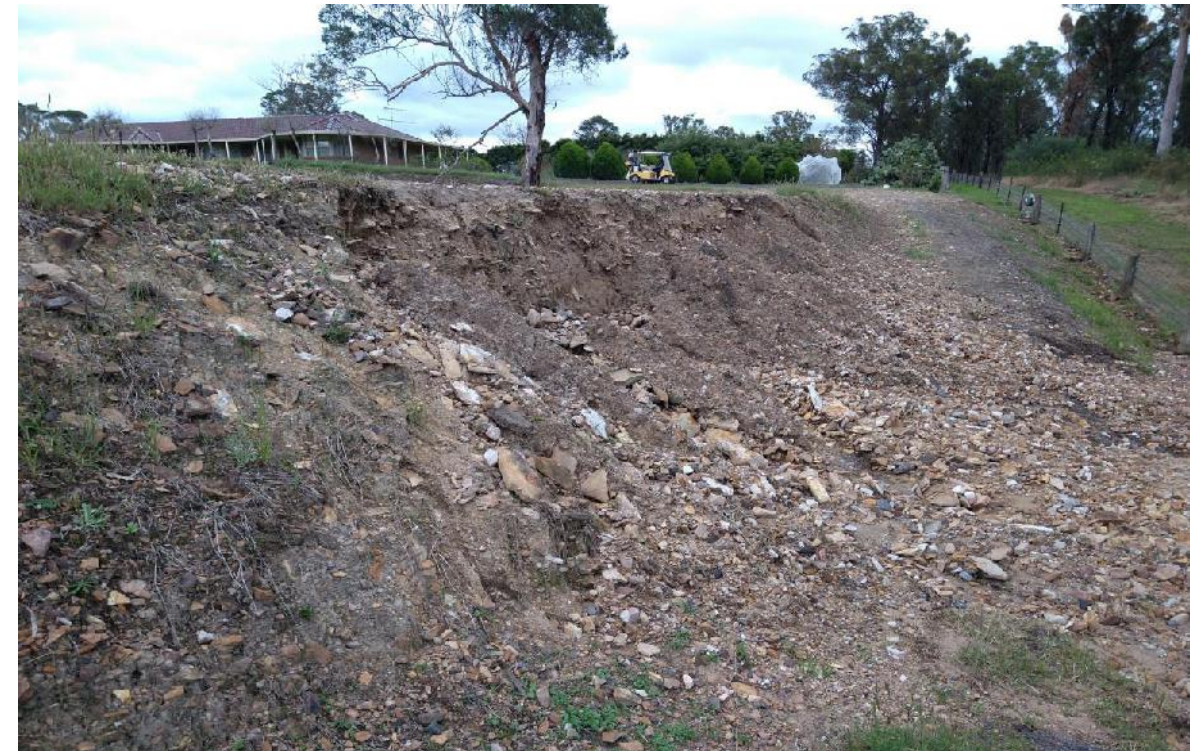
Photo 26: View looking west along the downstream toe of the farm dam at 4 Olive Lane (outside the SA). Note: the erosion and scour following overtopping during a heavy rainfall event in early April 2022.
