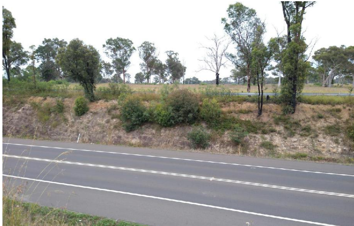
Photo 13: View looking southwest towards the road cutting adjacent to No. 3140 Remembrance Drive. Note: the soil and weathered rock in the upper cut and medium to thickly bedded rock in the
