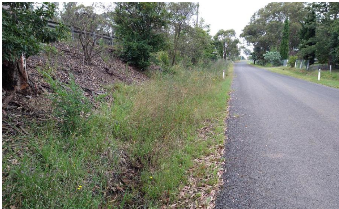
Photo 11: View looking south along the upstream face of RE4 opposite No. 3100 Remembrance Drive. Note: the drain cut into the toe of the embankment.
