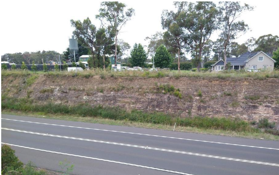
Photo 15: View looking east towards the cutting adjacent to No. 3165 Remembrance Drive. Note: the weathered rock in the upper cut and medium to thickly bedded rock in the middle and lower cut.
