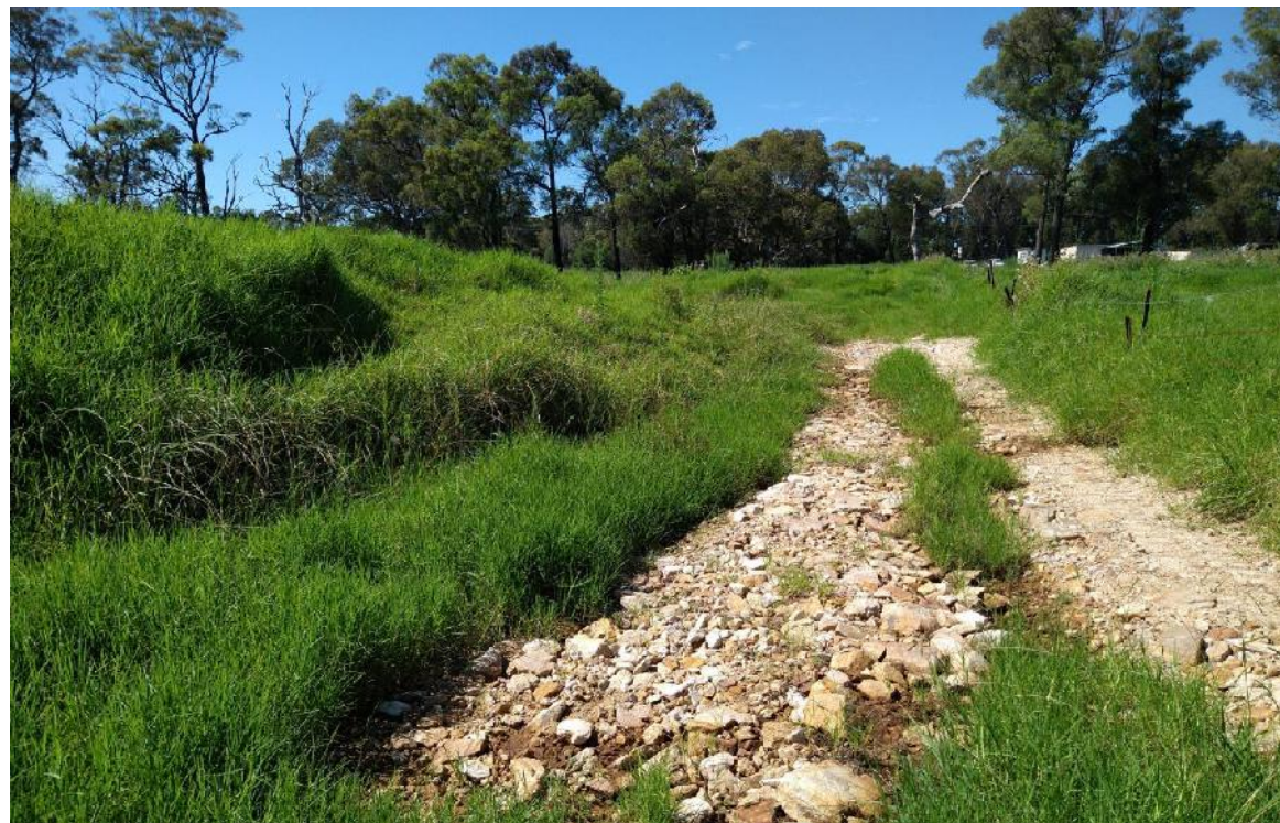
Photo 35: View looking along the spillway for FD15. Note: the embankment along the western side of the pond in the left of the photo.
