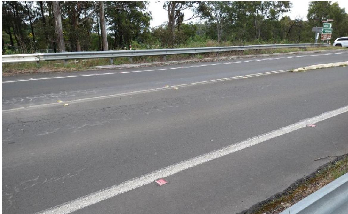
Photo 3: View looking north west at rutting and crocodile cracking in the Remembrance Drive wearing course to the south of the intersection with Wellers Road (RE1).
