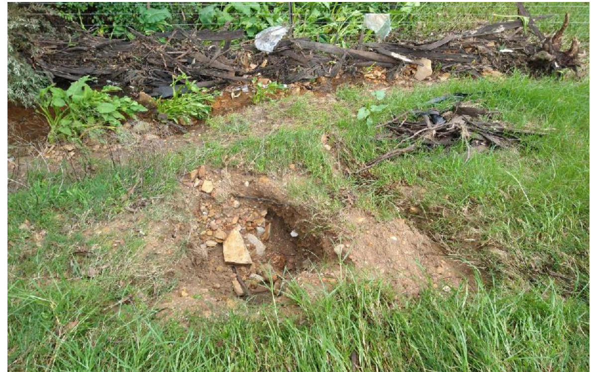
Photo 38: View looking at erosion and scour in the downstream face of FD27. Note the spillway channel at the toe of the embankment in the upper photo.
