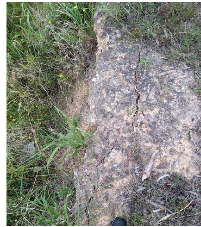
Photo 16: View looking at tension cracks setback behind the crest of opposite No. 3122 Remembrance Drive.
