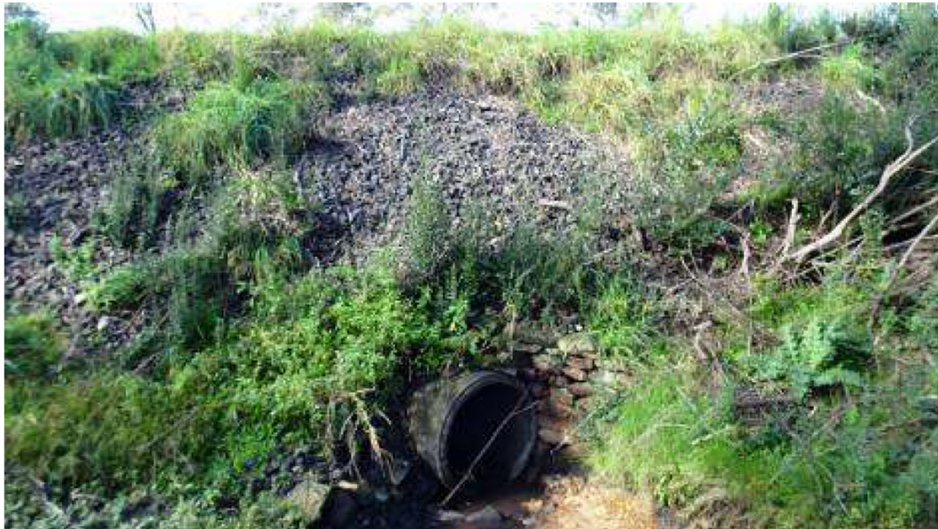
Photograph courtesy Newcastle Geotech
