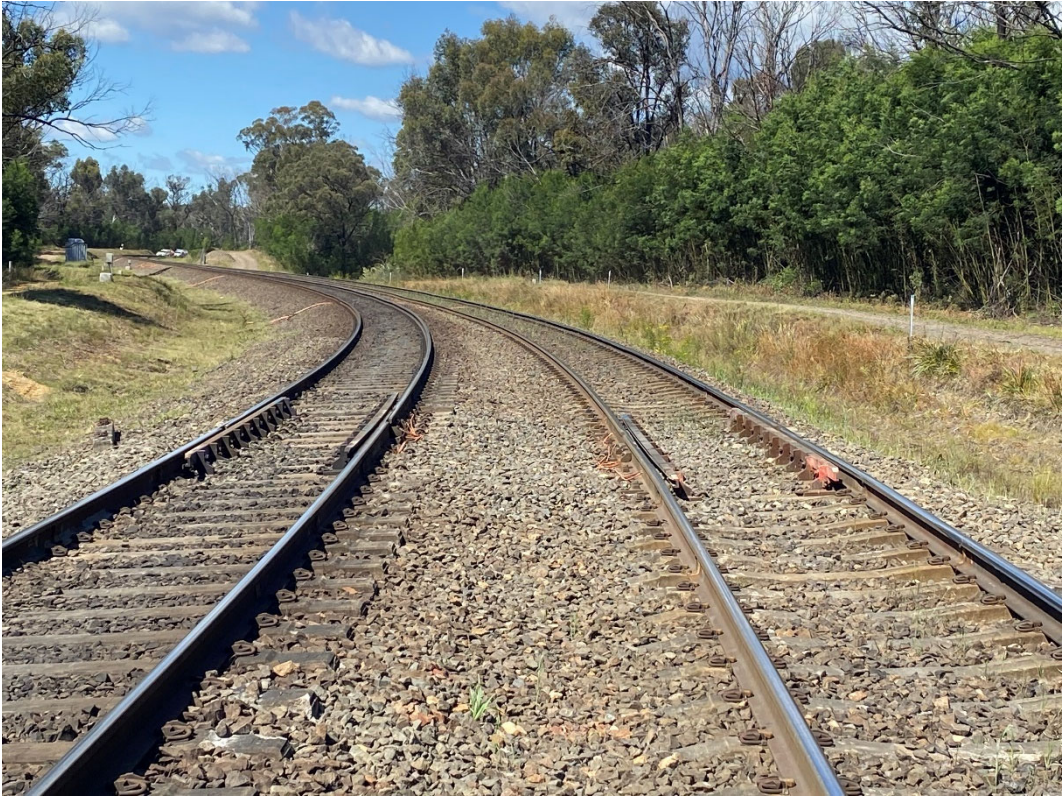
Fig. 3.5 Expansion switches installed at 98.560 km (ES2) prior to influence of LW S1A
