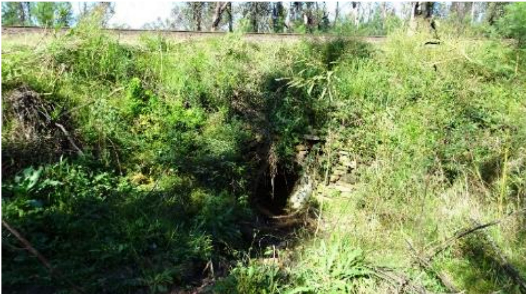
Photograph courtesy Newcastle Geotech
