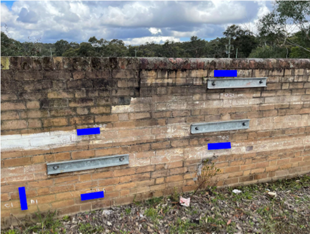
Photograph courtesy JMA Solutions (2022c) with blue lines where crack gauges are recommended
