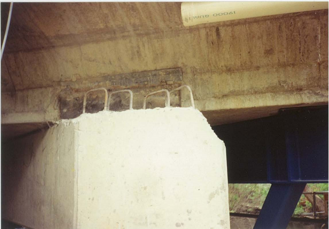
Fig. 3.40 Headstock bents / upstands removed at Rockford Road Bridge prior to mining of LW12
