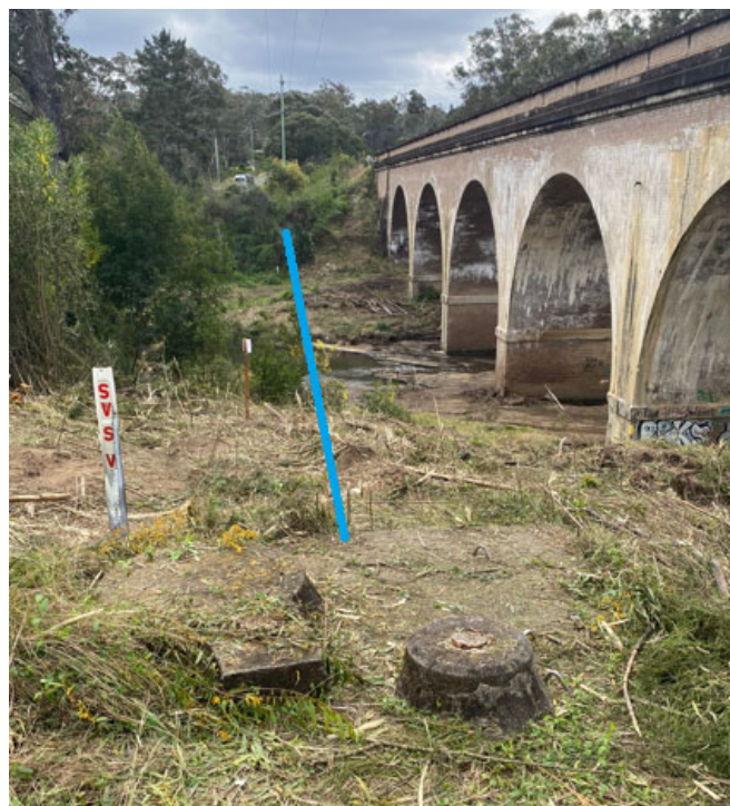
Fig. 3.16 Photograph of buried crossing of 450 mm CICL water main beneath the Bargo River adjacent to the Main Southern Railway Viaduct
