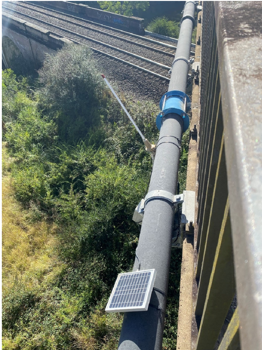
Fig. 3.7 150 mm DICL pressure main on Remembrance Drive Bridge over Bargo River
