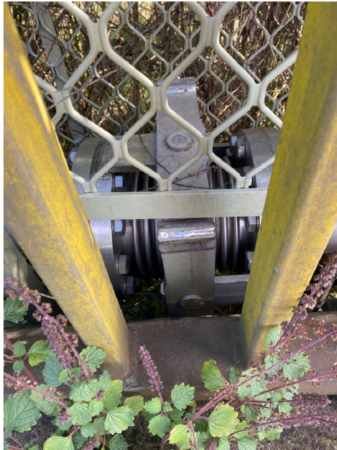
Fig. 3.9 Expansion joint for 150 mm DICL pressure main on Remembrance Drive Bridge over Bargo River
