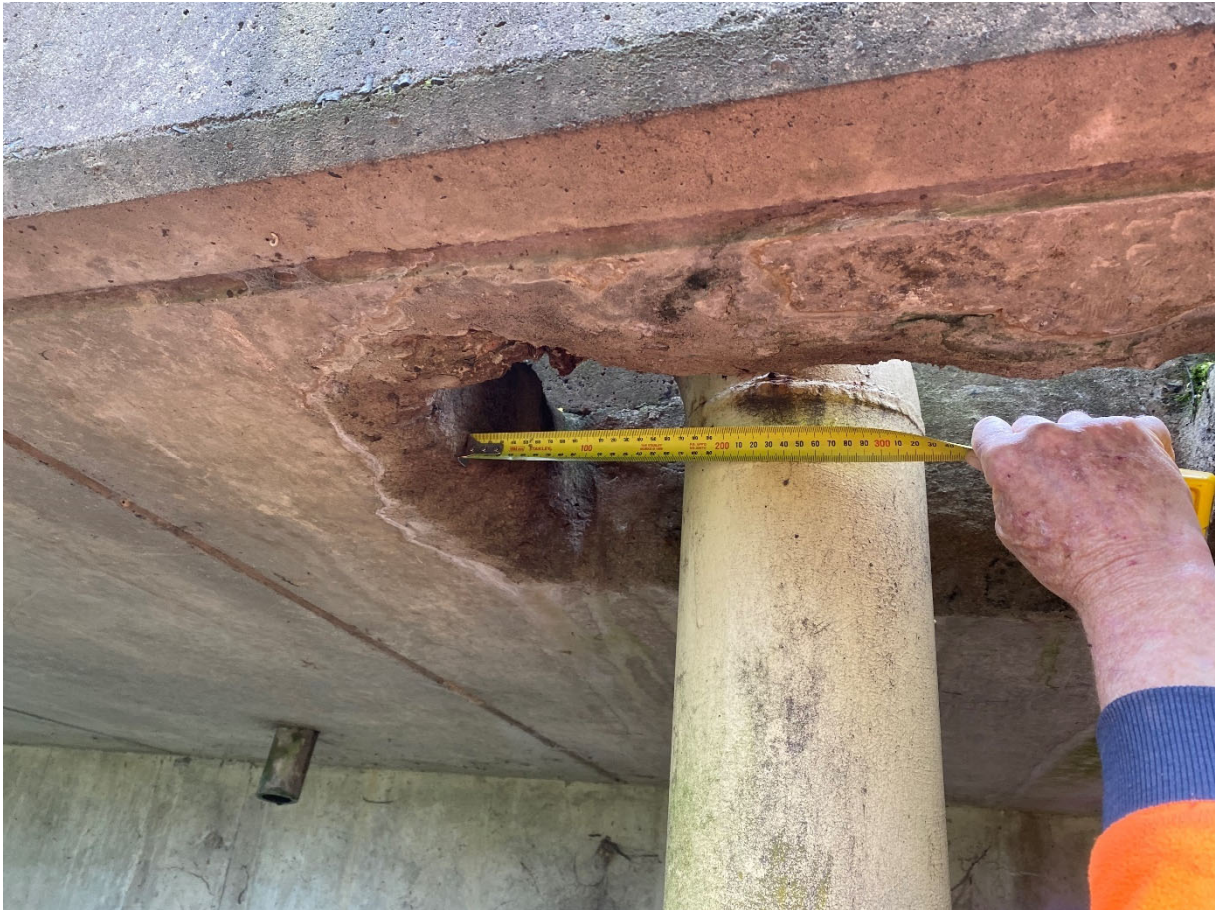
Fig. 3.18 Photograph of Jemena gas main pipe penetration for pipe bend on Remembrance Drive Bridge over the Bargo River
