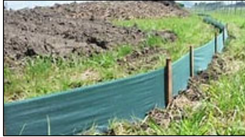
Figure 8 – Typical Sediment Control Fence
