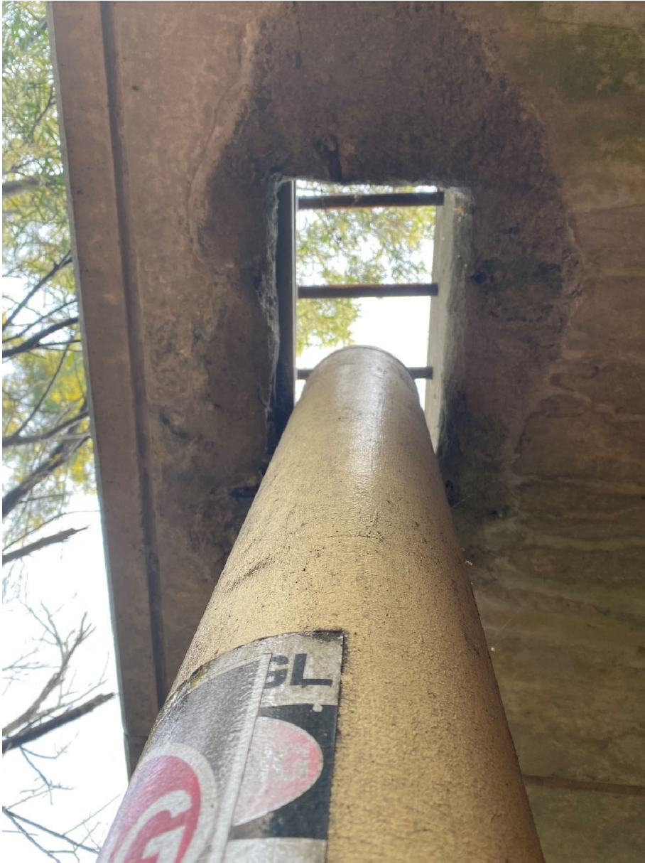
Fig. 3.17 Photograph of Jemena gas main vertical pipe bend on Remembrance Drive Bridge over the Bargo River
