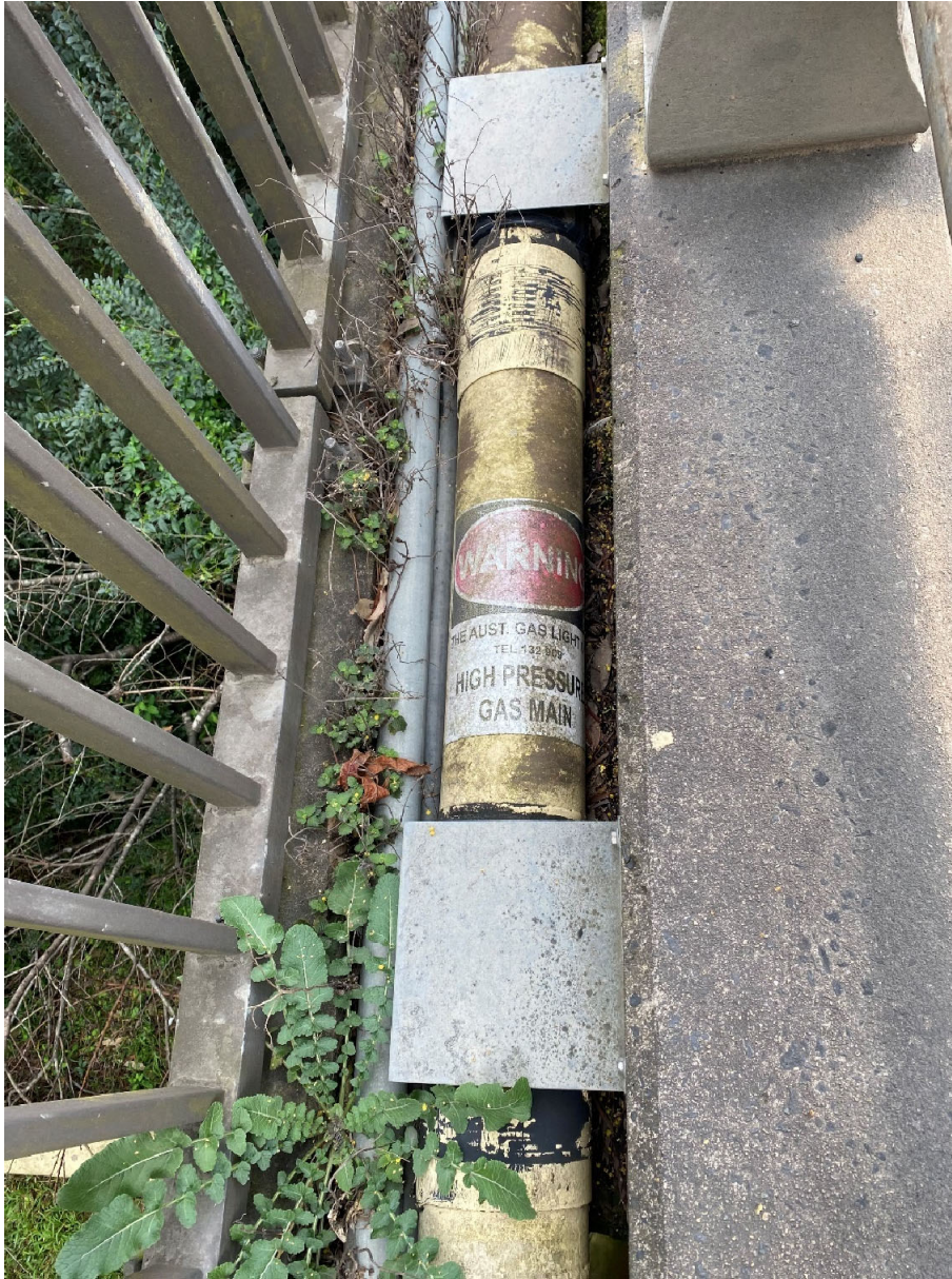
Fig. 3.16 Photograph of Jemena gas main on Remembrance Drive Bridge over the Bargo River
