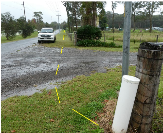
Plate 7: View north along Great Southern Rd towards Charlies Point Rd showing Telstra P35 conduit route containing NBN cable
