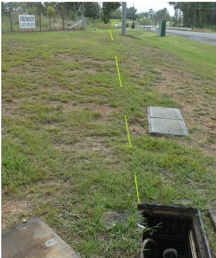
Plate 3: Telstra pit on north side of Yarran Road over LW S5A, showing route of NBN IEN cable 2-TAH-0300-DSS-005 along western side of Remembrance Drive and crossing LW S5A north to LW S1A
