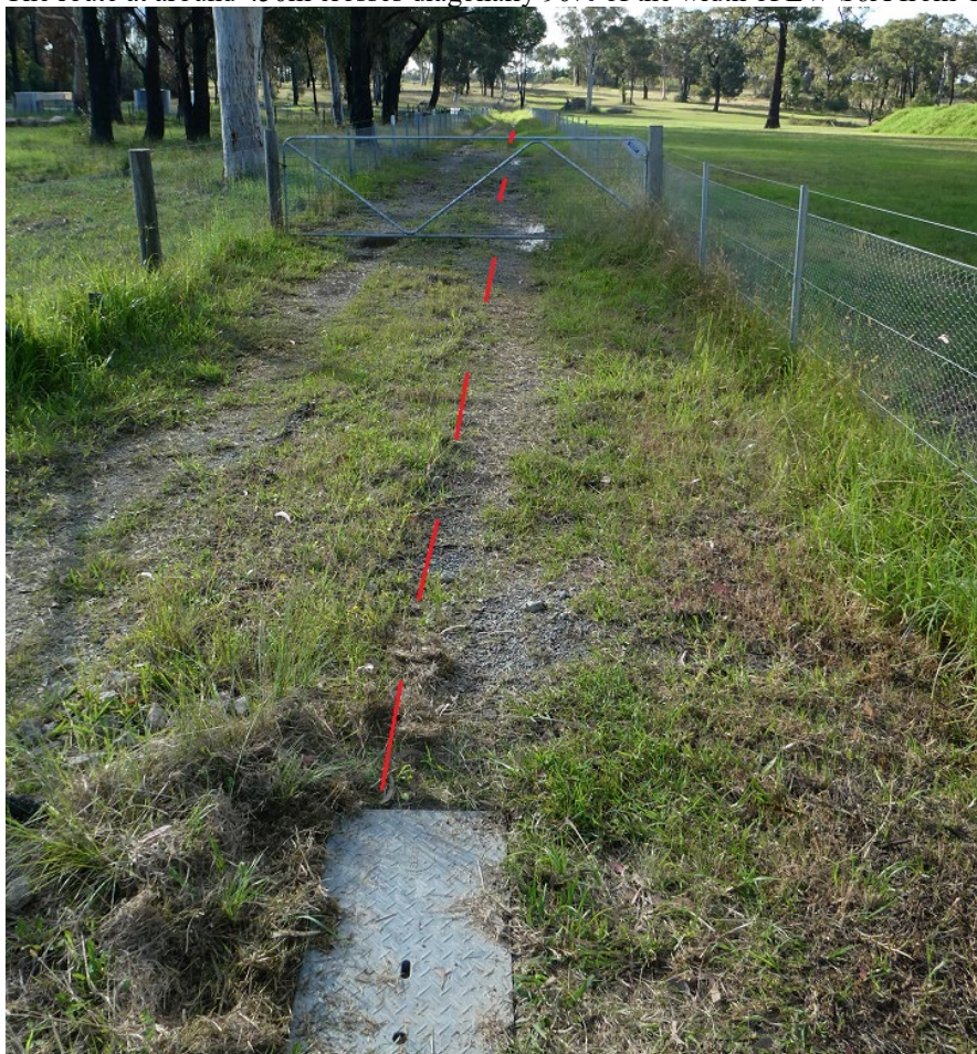
Plate 6: View north from Yarran Road entry to tower site. Shows approx. location of buried underground power supply to the site from pole in Yarran Road. Note the Power Line also crosses a shallow creek line along the access track and above the centerline of LW S6A.
