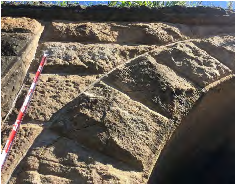
Eastern portal. No worsening of cracking during extraction of LW W3.
