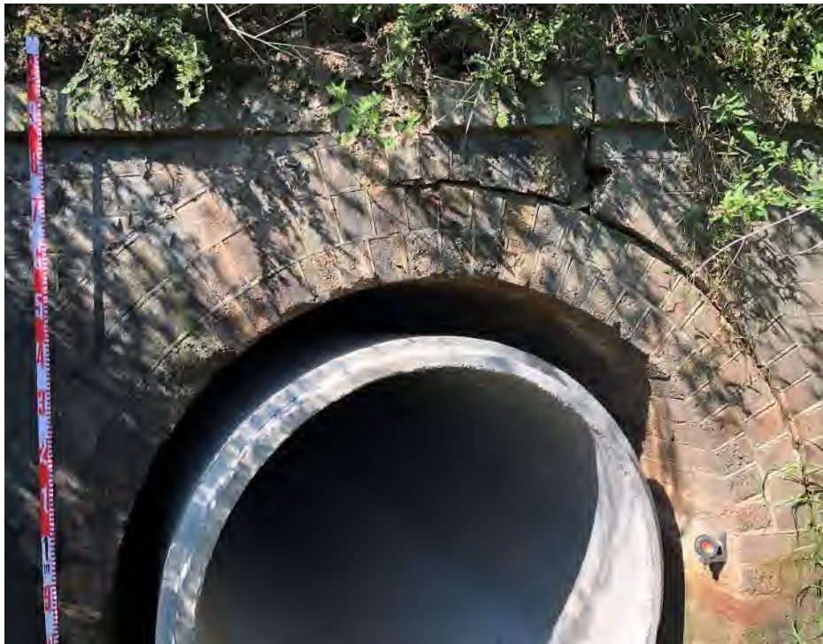
Cracking and displacement of bricks around the western portal arch. Does not appear to have worsened during longwall mining in the Western Domain.
