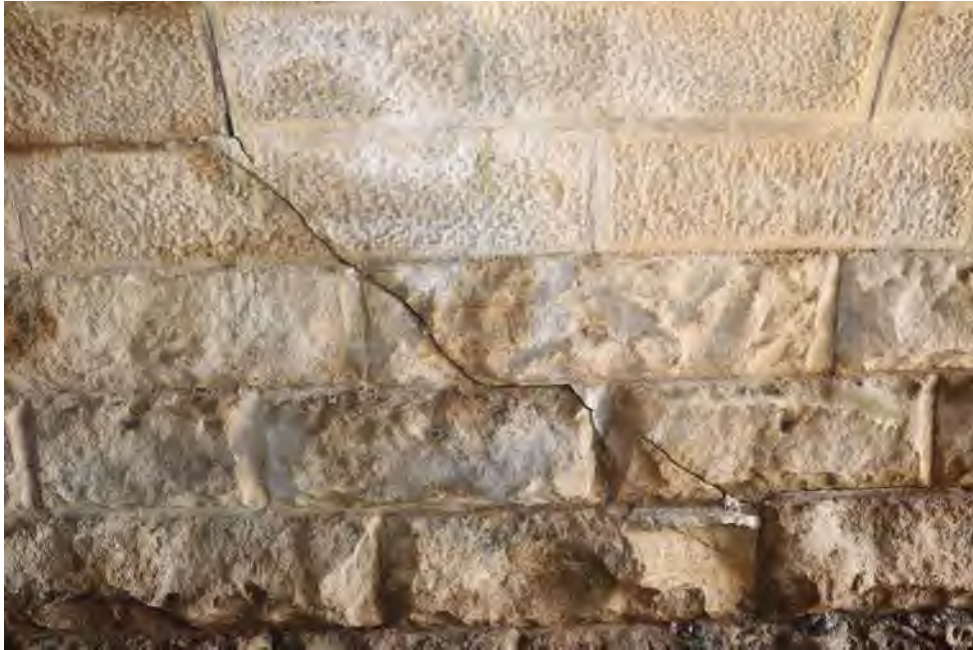
Photo 88.400-7 Identified crack 3 to culvert barrel. Not noted in the pre-mining report.
