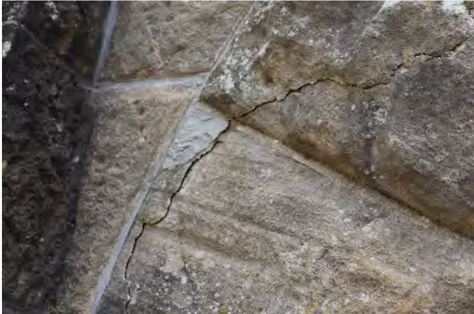
Photo 88.400-3 Eastern portal. No worsening of cracking during extraction of LW W4.
