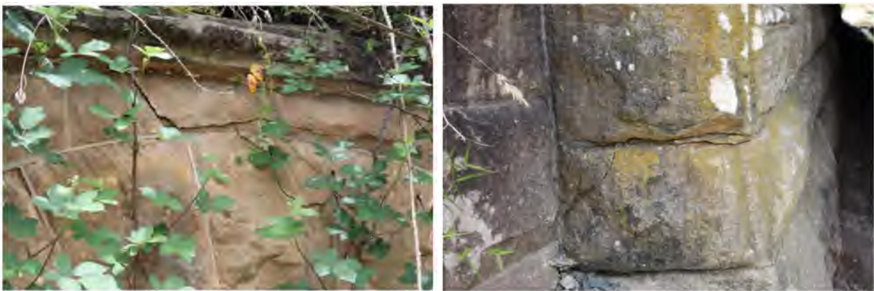
Figure 3-1 Cracking on the portal ends at culvert 88.400 km. This cracking has not worsened during the mining of LW W4.
