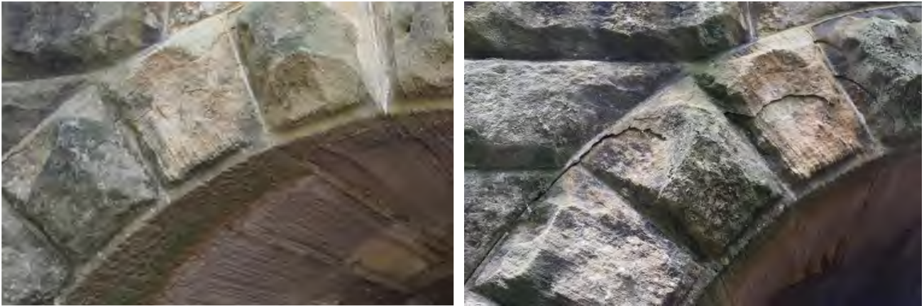
Photo 88.980-2 Western portal. Pre-mining (left) and post-mining (right) inspection photographs. Cracking along the mortar and spalling of the arch stones has not worsened significantly during extraction of LW W4.
