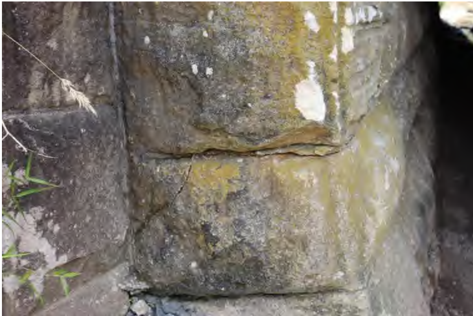
Photo 88.400-4 Eastern portal. Cracking to the arch of the culvert previously identified has not worsened significantly during LW W4.
