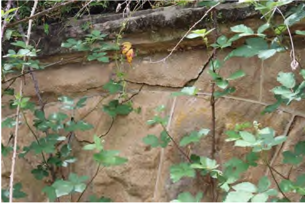
Photo 88.400-1-Western portal. Spalling above the arch that developed during extraction of LW W2 has not worsened significantly during LW W4.
