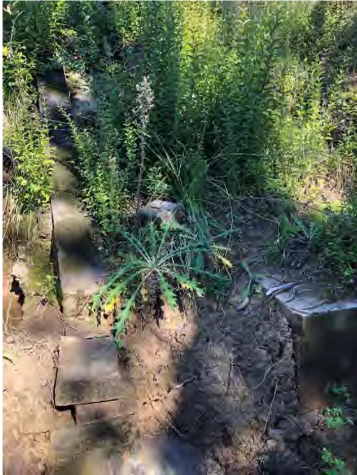
Photo 87.330-2 Displaced bricks at the base of the brick chute to the south of the eastern portal.
