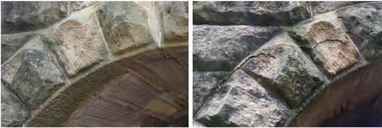
Figure 3-3 Cracking at culvert 88.980 km. Pre-mining (left) and post-mining (right) inspection photographs. Cracking along the mortar and spalling of the arch stones has not worsened significantly during extraction of LW W4.
