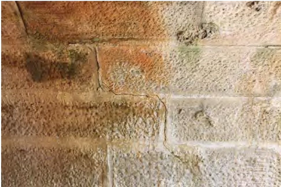
Photo 88.400-8 Identified crack 4 to culvert barrel. Not noted in the pre-mining report.
