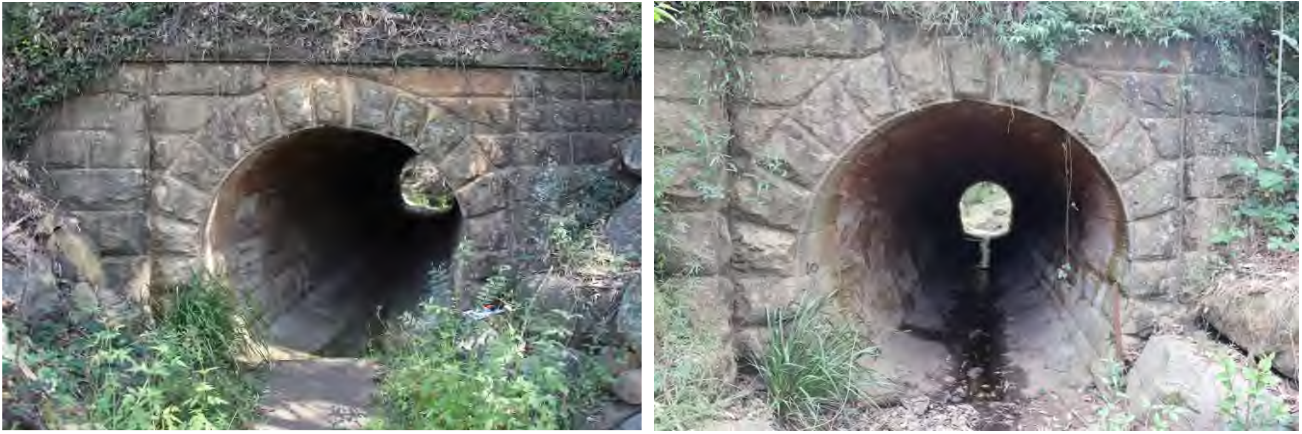
Photo 88.980-5 Eastern portal. Pre-mining (left) and post-mining (right) inspection photographs. Generally in good condition with no new cracking due to extraction of LW W4.
