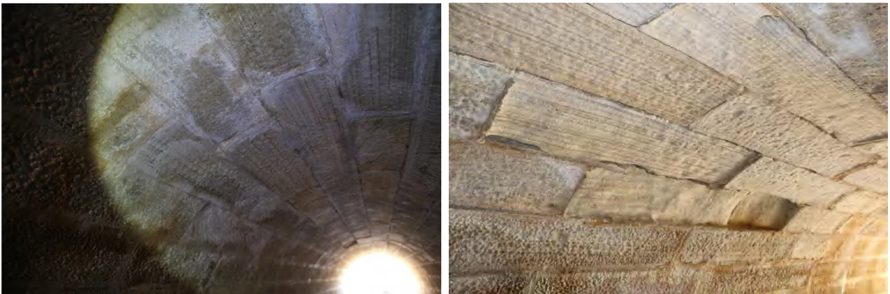
Photo 88.400-9. Pre-mining (left) and post-mining (right) inspection photographs. Isolated section of sandston erosion towards western portal. Not noted in the pre-mining report however no noted increase in surface erosion during LW W4.
