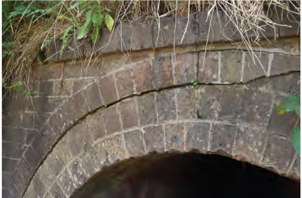
Photo 87.850-2 Detail, pre-existing cracking and displacement of bricks around the eastern portal arch that does not appear to have worsened significantly during longwall mining in the Western Domain.
