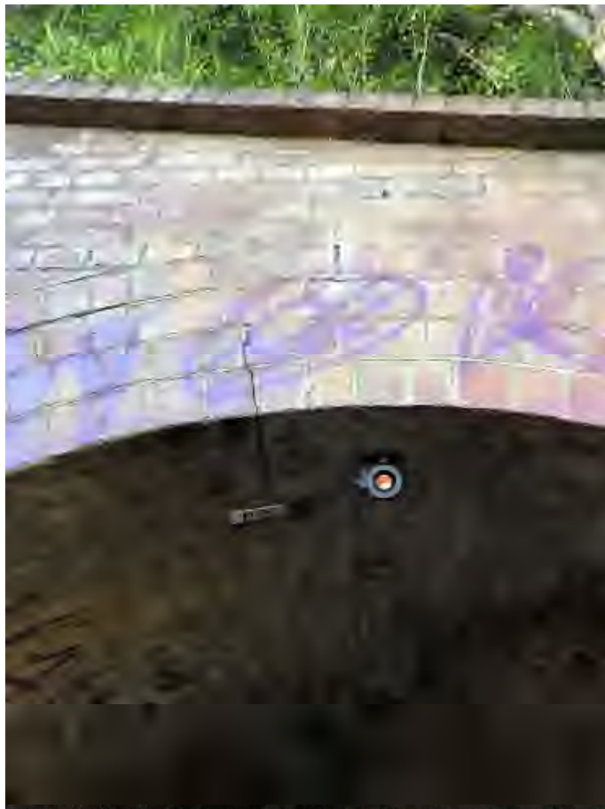
Western portal. Cracking through the mortar above the arch continues along the roof of the culvert.
