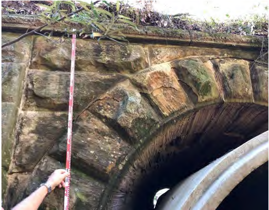
Western portal. Cracking along the mortar and spalling of the arch stones has not worsened significantly during extraction of LW W3.
