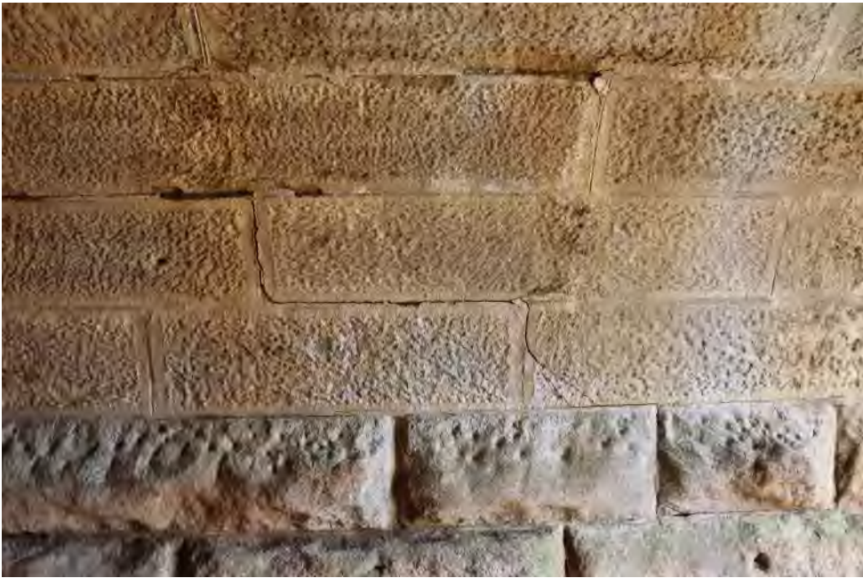
Photo 88.400-6 Identified crack 2 to culvert barrel. Not noted in the pre-mining report.
