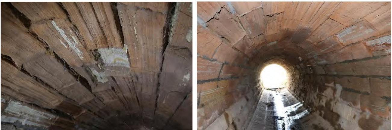
Photo 88.980-3 Barrel of culvert. Pre-mining (left) and post-mining (right) inspection photographs. Significant surface erosion and exfoliation throughout the barrel noted in the pre-mining report.
