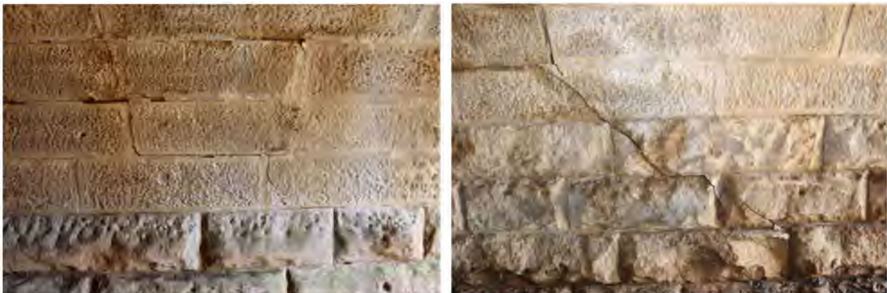
Figure 3-2 Cracking in the barrel of culvert 88.400 km. This cracking has formed during the mining of the Western Domain.
