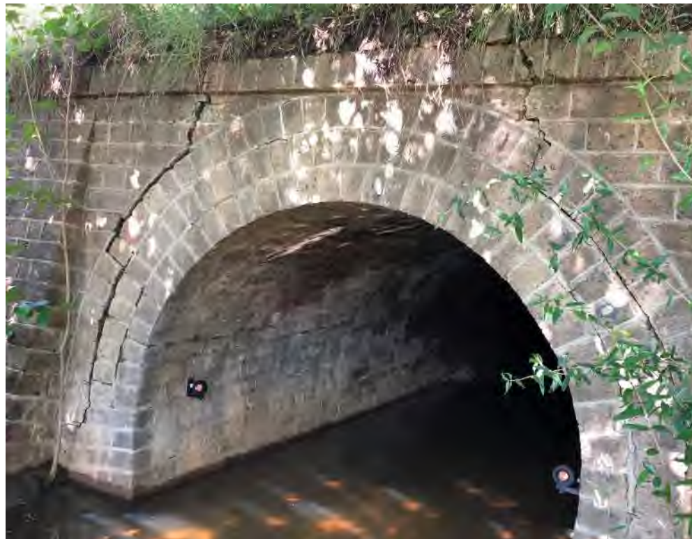
Photo 87.300-1 Northern portal. Difficult to access due to water and weeds. Pre-existing cracking around the arch, mostly through mortar.
