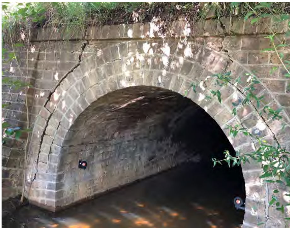
Northern portal. Difficult to access due to water and weeds. Pre-existing cracking around the arch, mostly through mortar.
