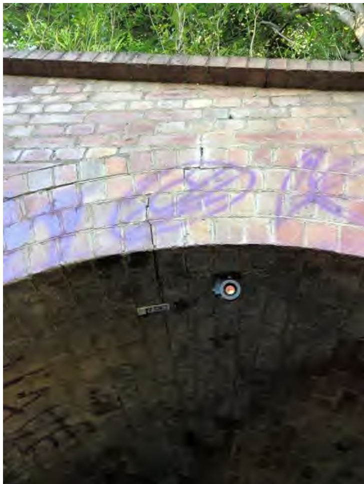
Photo 89.216-3 Western portal. Cracking through the mortar above the arch continues along the roof of the culvert.
