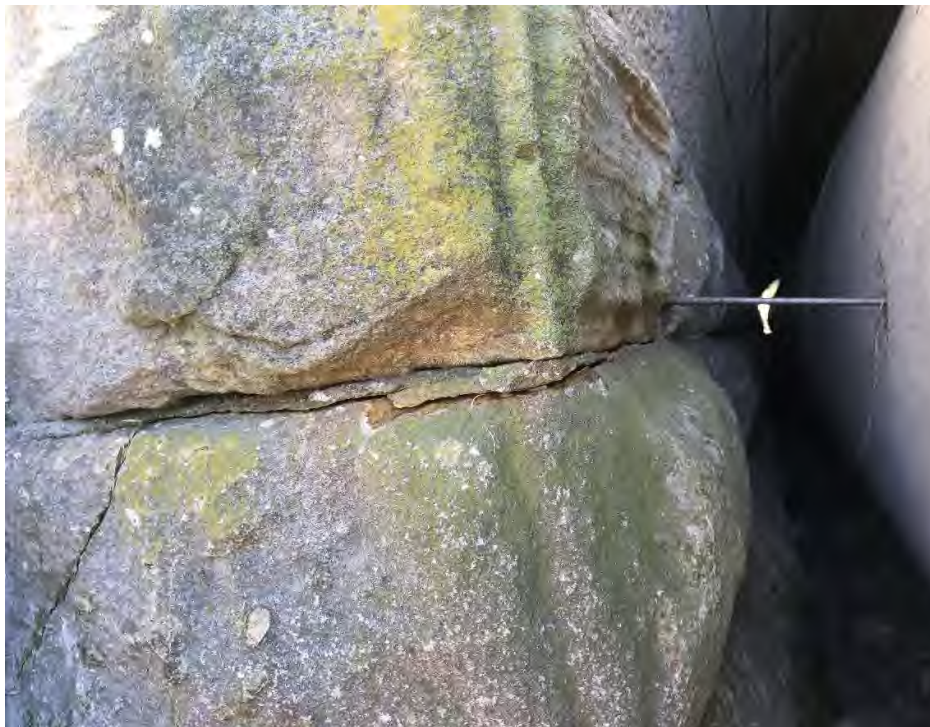
Eastern portal. Screw securing concrete sleeve to the arch of the culvert has resulted in some cracking along the mortar and through the sandstone.
