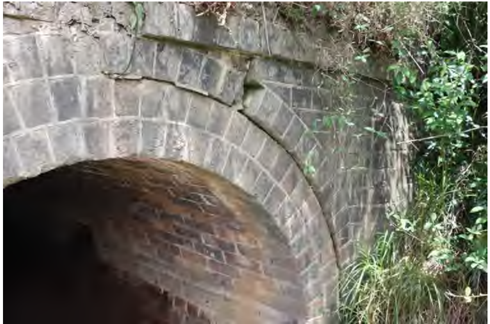
Photo 87.850-4 Cracking and displacement of bricks around the western portal arch. Does not appear to have worsened during longwall mining in the Western Domain.
