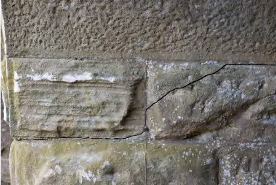
Photo 88.400-5 Identified crack 1 to culvert barrel. Not noted in the pre-mining report.
