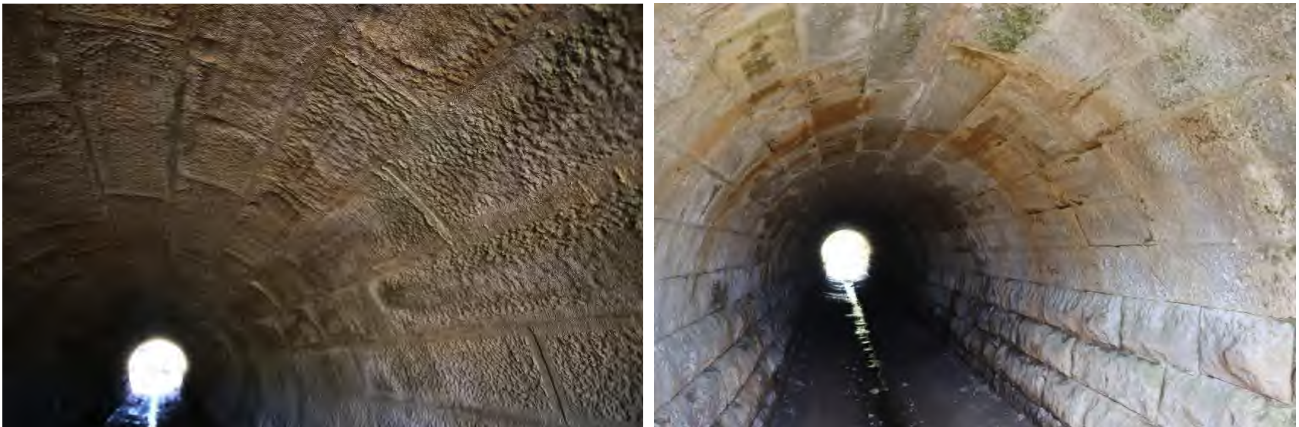
Photo 88.400-2 Barrel of culvert. Pre-mining (left) and post-mining (right) inspection photographs. In generally good condition with only minor cracking to sandstone blocks.
