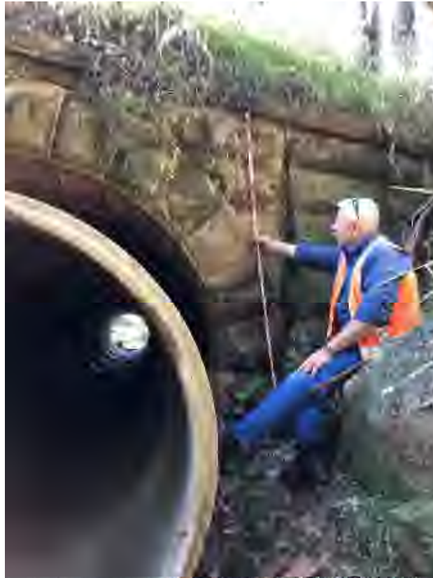
Western portal. Cracking around arch stones that was first noted during extraction of LW W2 has not worsened during LW W3.
