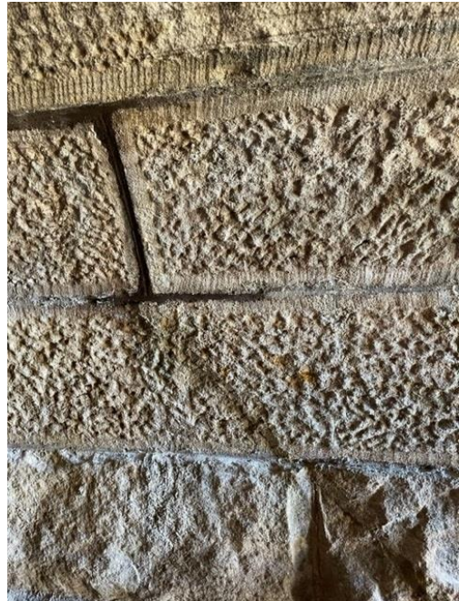
Figure 3: Crack and mortar repairs
