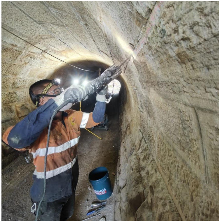
3. Route cracked mortar beds
