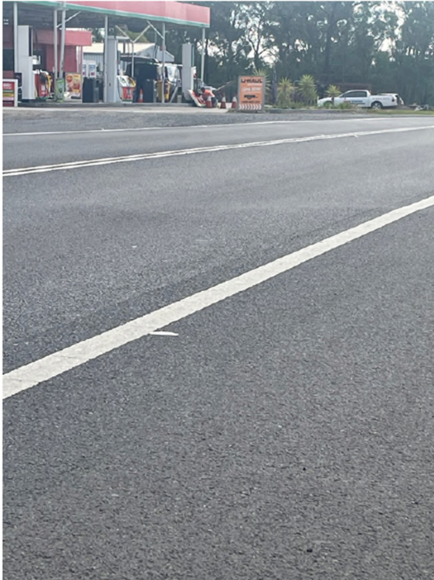
Figure 2-19 Small bump observed in southbound lane of Remembrance Drive near Peg R46 on 31 May 2023 (Source: MSEC1304 Report 38, Appendix A)
