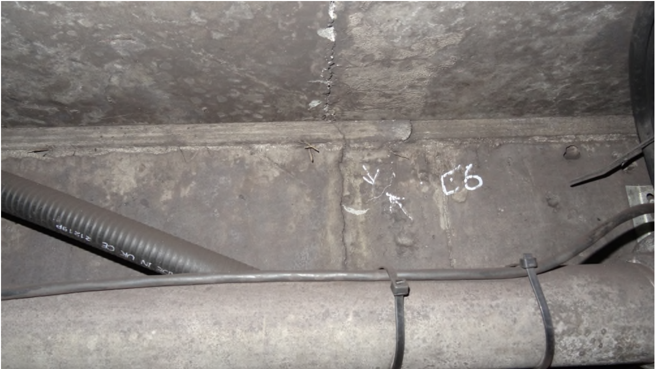
Photo 6: General location of crack C6.
