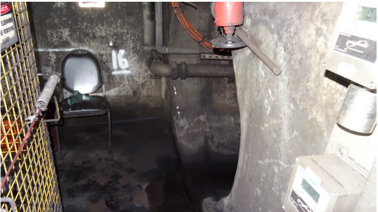
Photo 3: General location of cracks C1 and C3.
