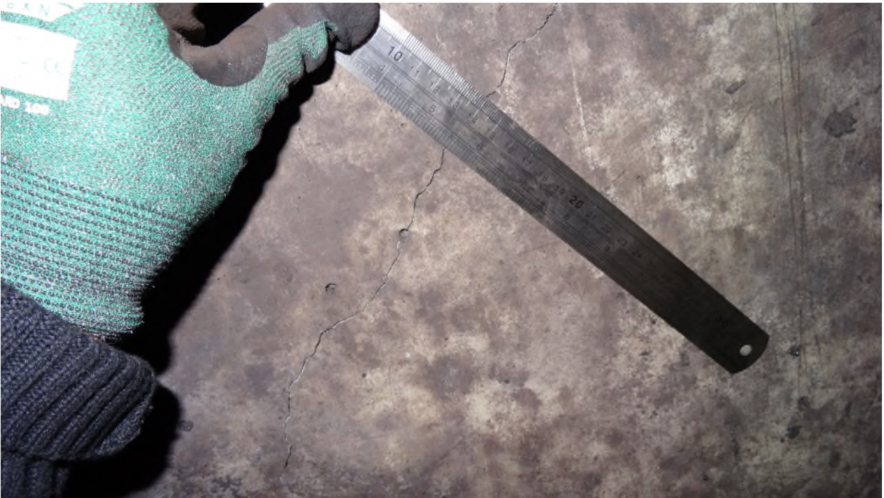
Photo 5: Crack B showing crack width < 1\text{mm} .
