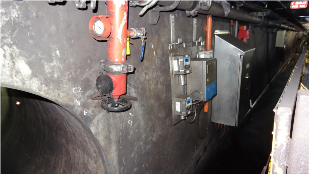
Photo 2: General location of cracks C2 and C3.
