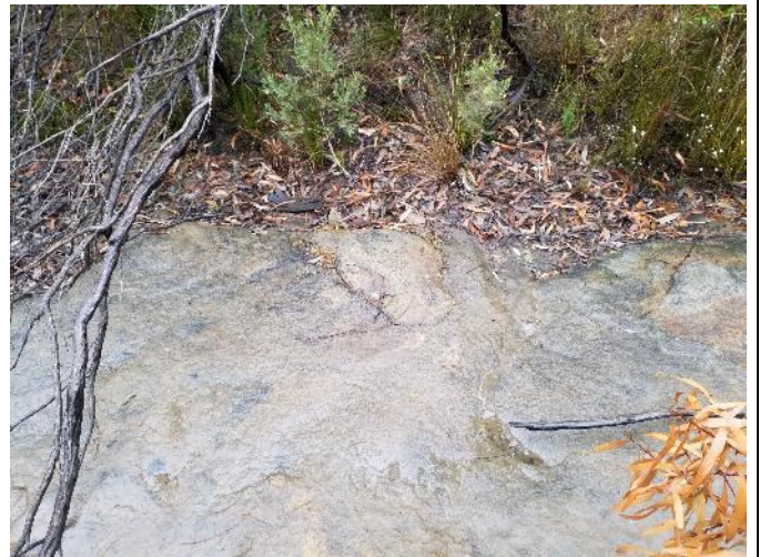
Cracking on South bank of Rockbar 2 28/06/2023
