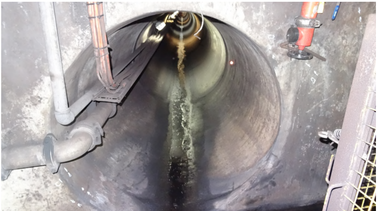
Photo 1: General location of cracks C1, C2 and C3.
