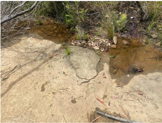
Cracking on South bank of Rockbar 2 15/11/2022
