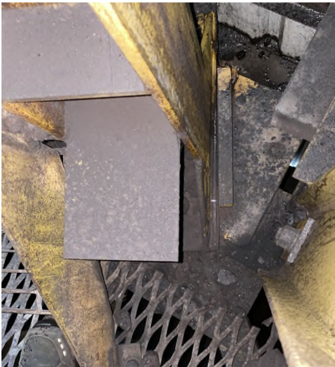
Figure 2: 7C slide joint west (22/05)
