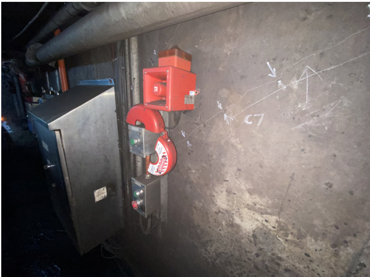
Photo 3: Location of new crack (C7).
