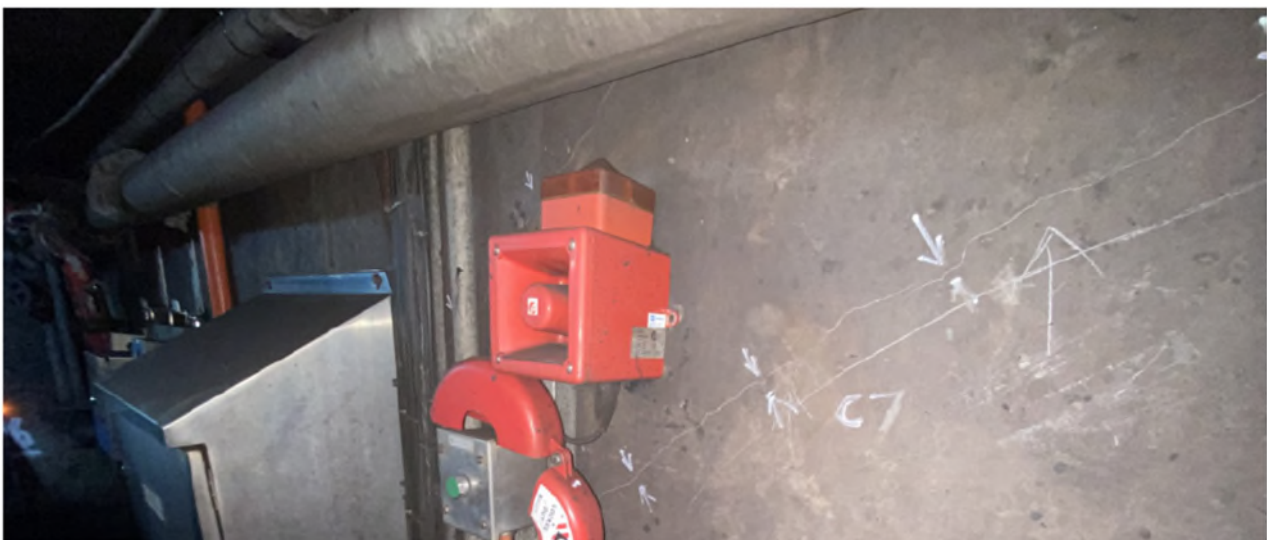
Figure 2-20 Schematic of cracks located in 6C Tunnel and example of crack (crack C7 taken 27 June 2023) (Source: Photo report: Tahmoor Mine Conveyors 27/9/2023, Appendix G)
