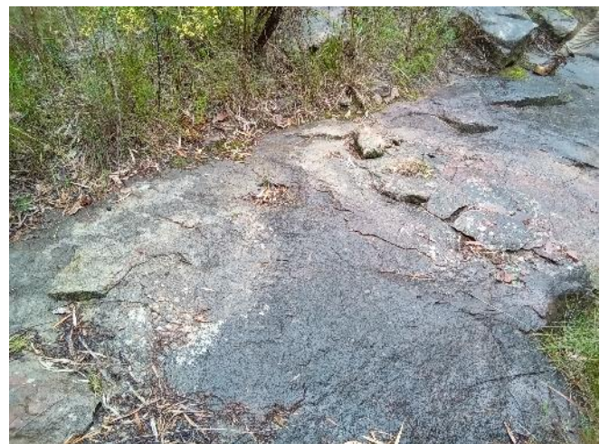
Additional Photo Cracking upstream 28/06/2023
