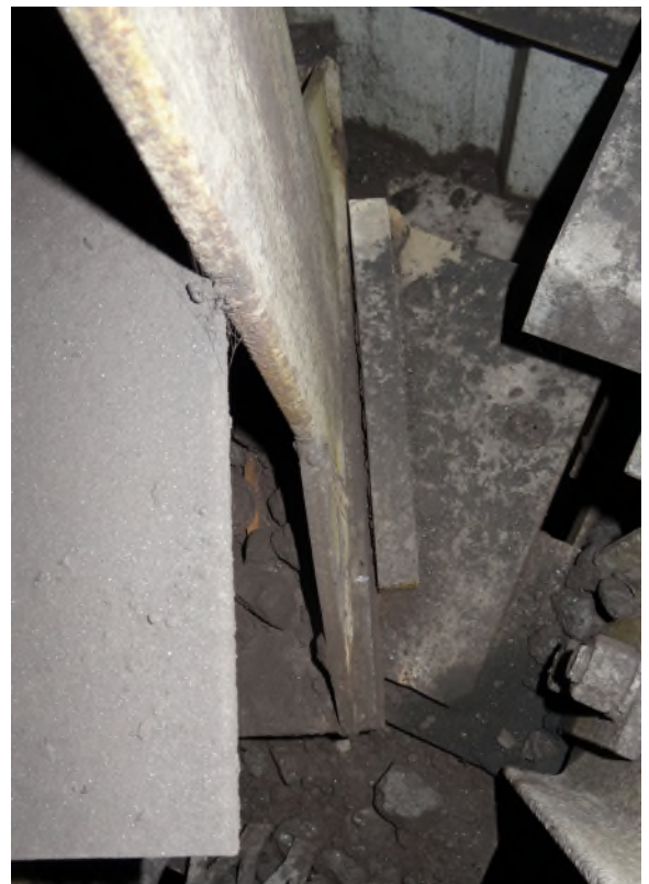
Figure 3: 7C slide joint west (29/05)
