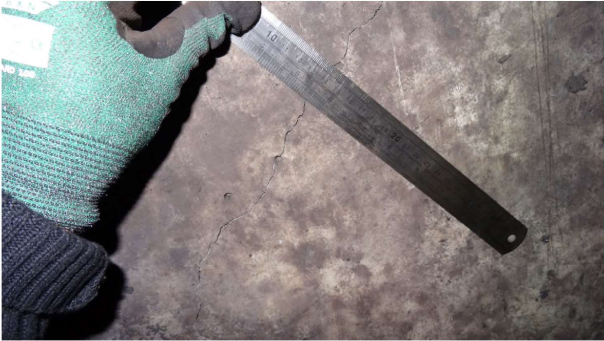
Plate 4.2 Crack B (C2), width <1 mm (David Talbert 29 May 2023).
