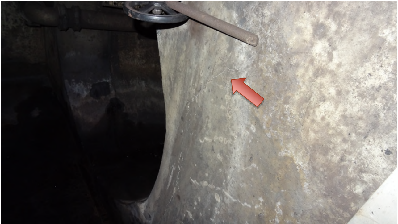
Photo 3: Crack B at edge of vent shaft tunnel extending toward roof.
