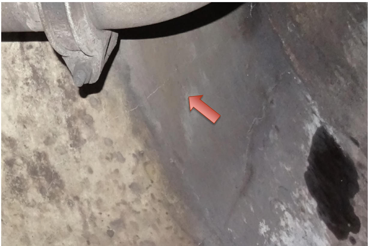
Photo 2: evidence of finer cracking above larger crack.
