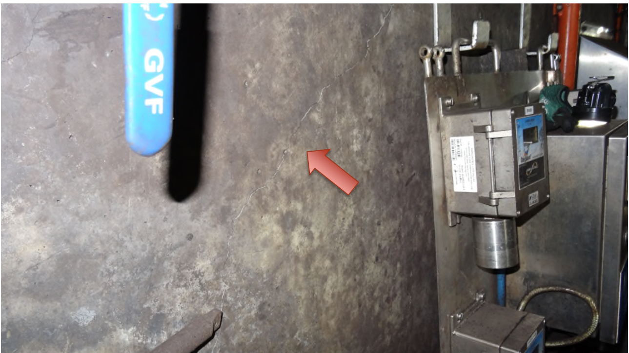
Photo 4: Crack B extending toward 6C tunnel roof.
