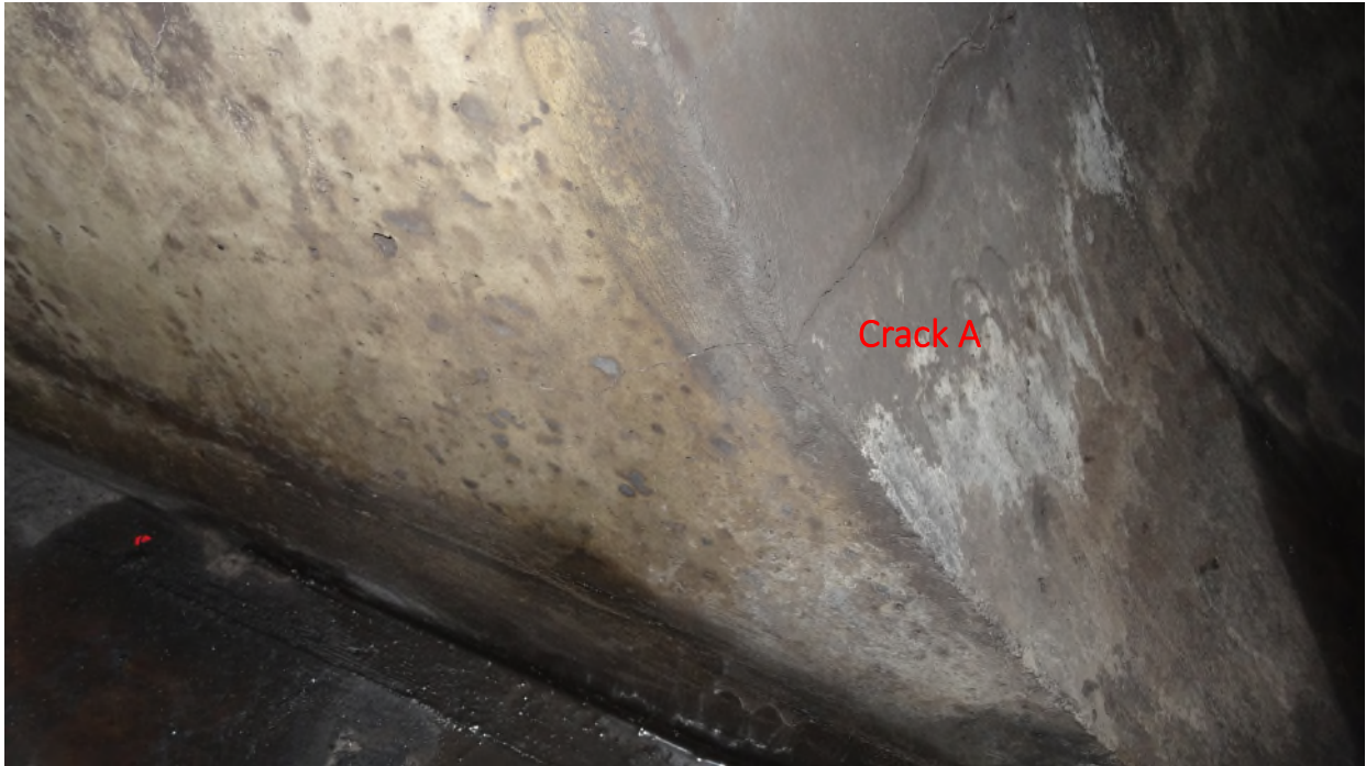
Photo 1: Crack A located approximately 7 O'clock along western face extending into the vent shaft tunnel.
