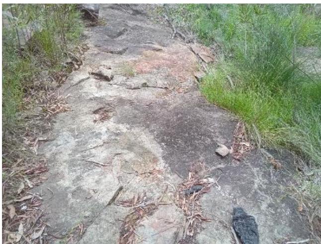
Additional Photo Cracking upstream 08/02/2023
