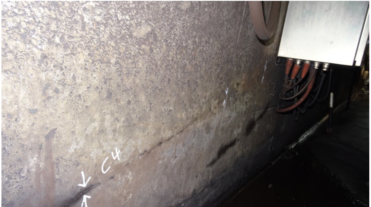
Photo 4: General location of cracks C4.
