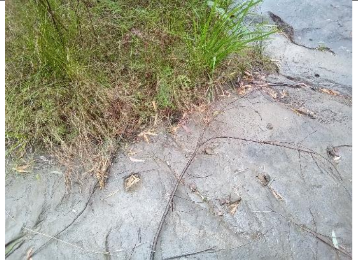
Additional photo Iron Staining 28/06/2023
