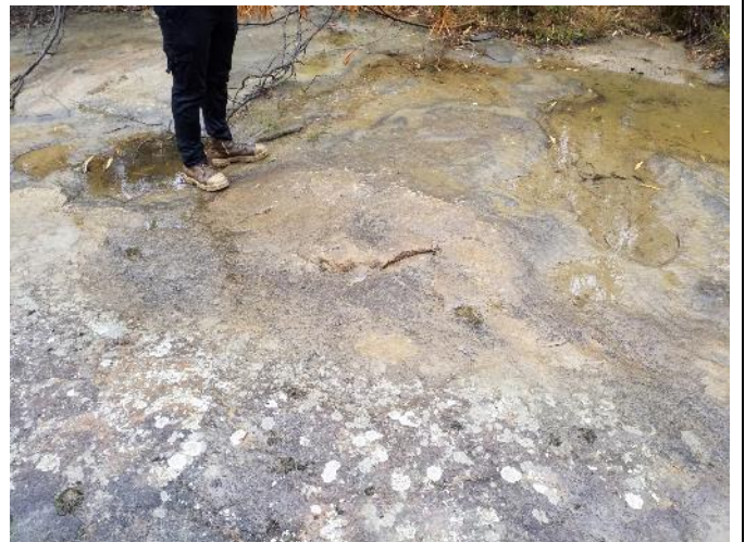
Weathering, cracking on North bank of Rockbar 2 28/06/2023
