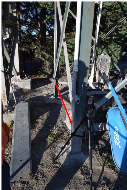
Figure 3 Location of missing angle tie indicated by red double-headed arrow.
