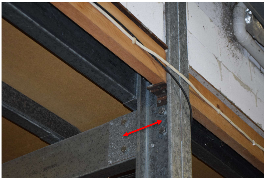
Figure 5 Back-to-back steel columns continue up to support the high-bay roof and are effectively restrained by the Hebel blockwork in the minor-axis direction, major-axis load eccentricity indicated by red arrow.
