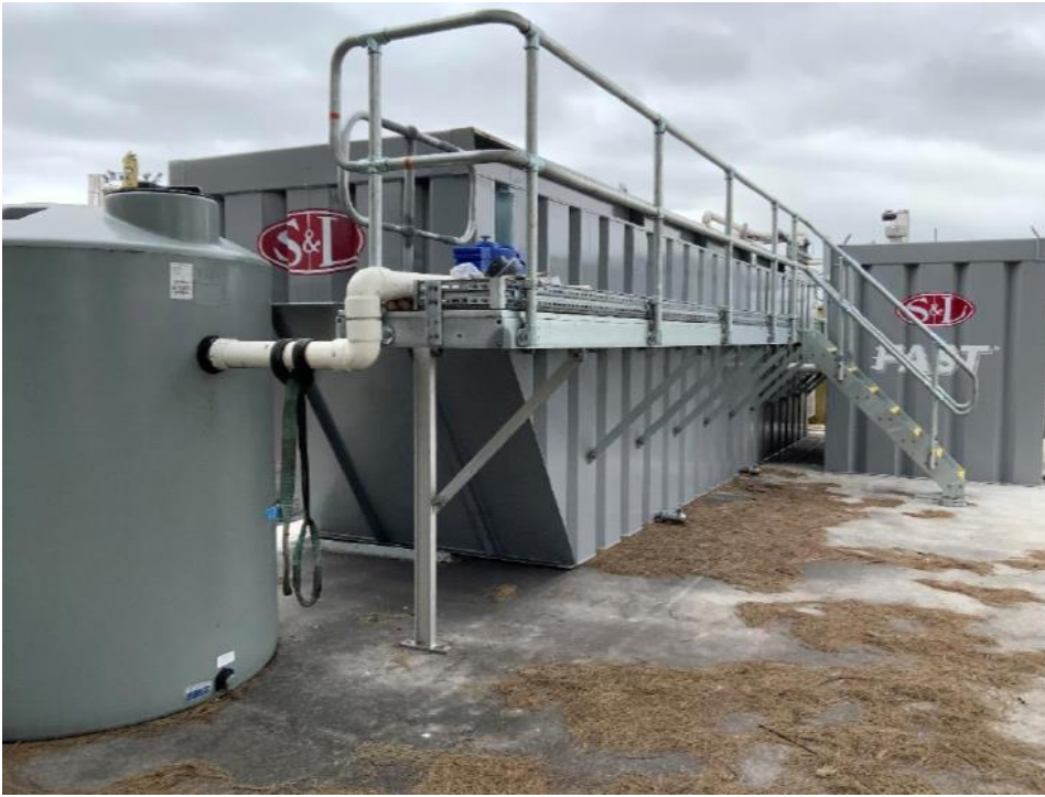
Figure 10: Smith & Loveless Sewage Treatment Plant (STP) onsite
