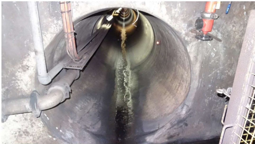
Plate 4.3 Context for the location of cracks C1, C2 and C3 (David Talbert, 6 June 2023).
