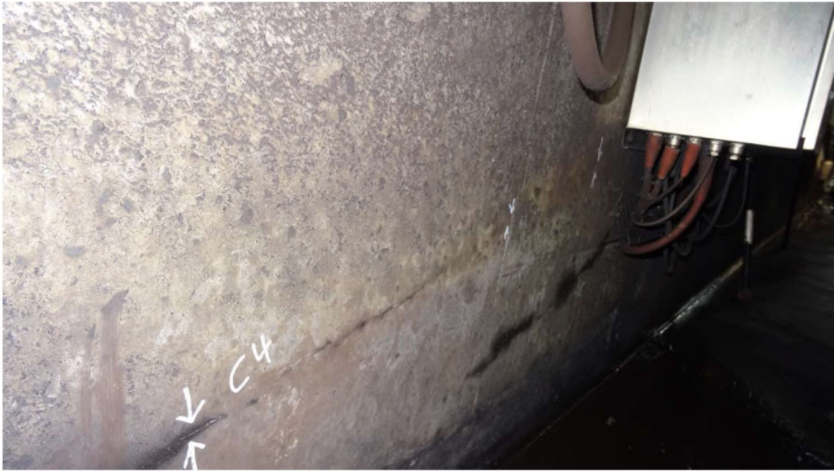
Plate 4.4 Crack C4 (David Talbert, 6 June 2023).
