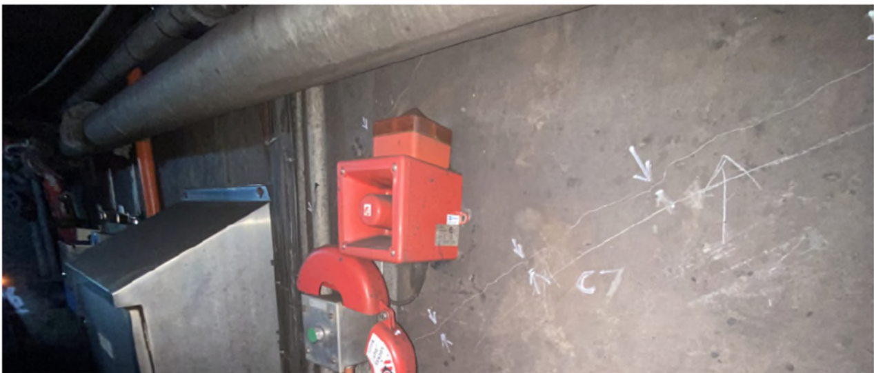
Figure 3-20 Schematic of cracks located in 6C Tunnel and example of crack (crack C7 taken 27 June 2023) (Source: Photo report: Tahmoor Mine Conveyors 27/9/2023, Appendix F)
