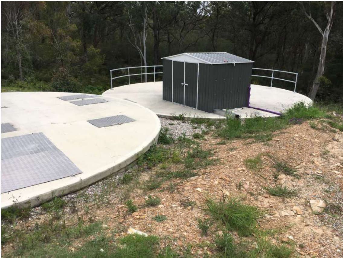
Fig. 7.11 Wollondilly Anglican College – Sewage treatment tanks
