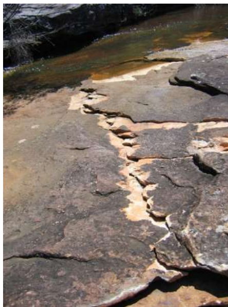
Fig. 4.12 Surface tension cracking along the top of a steep slope
