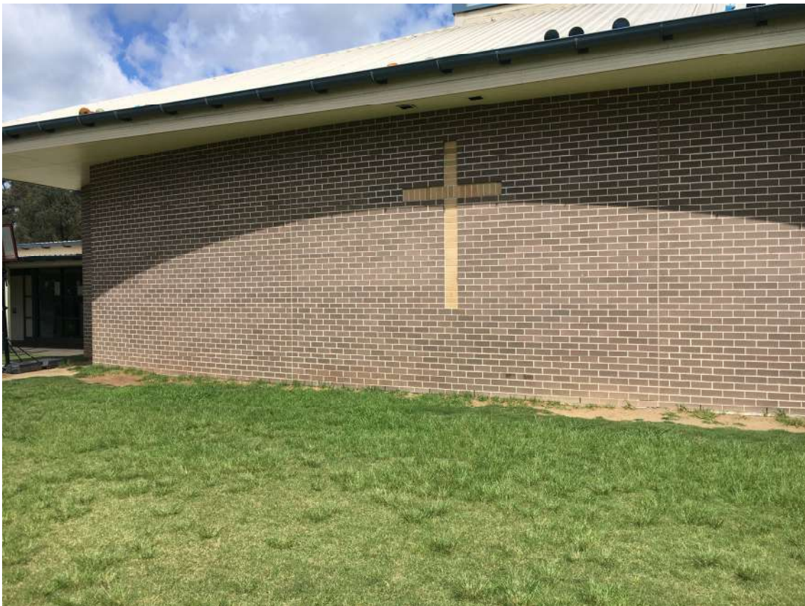
Fig. 7.2 Wollondilly Anglican College – Clifford Warne Auditorium with articulation joints in brick wall
