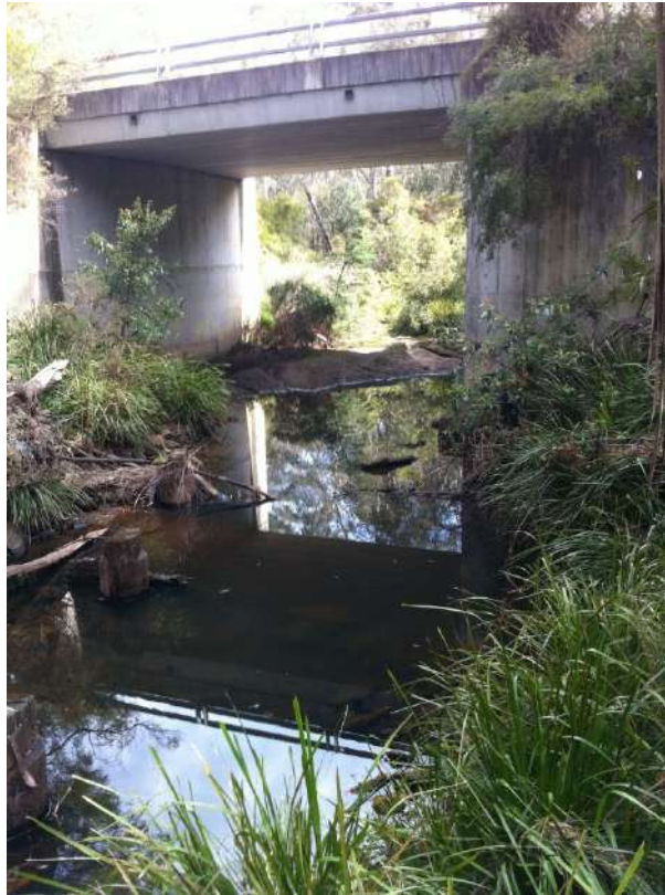
Fig. 5.8 Ponded water in Dog Trap Creek near bridge over Arina Road above previously extracted Longwall 13
