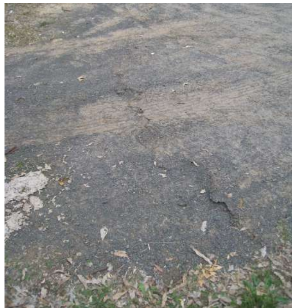
Fig. 4.10 Surface compression buckling observed in a pavement
