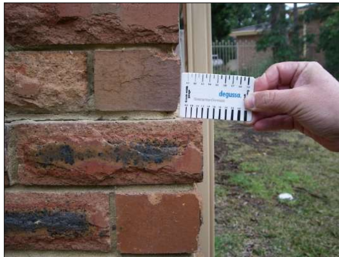
Fig. C.1 Example of slippage on damp proof course
