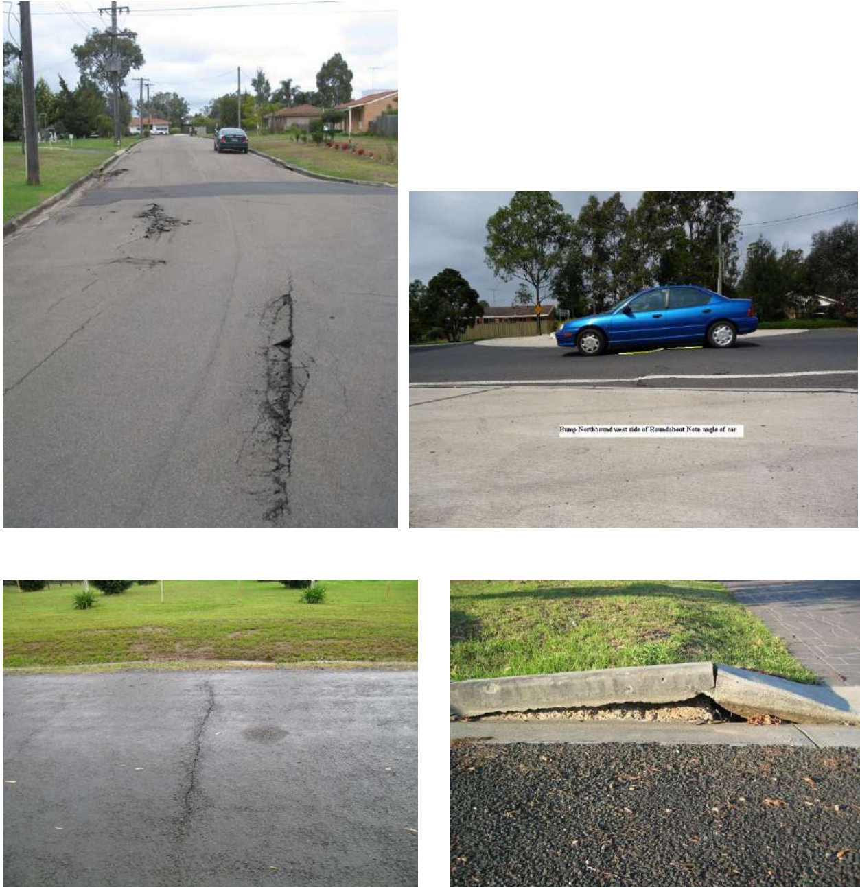
Fig. 6.20 Previously observed impacts on local roads above Tahmoor Mine
