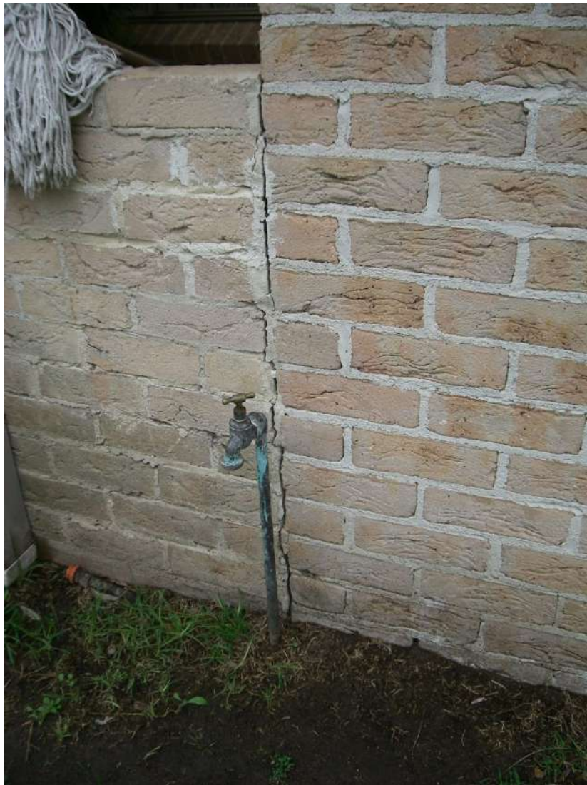
Fig. C.2 Example of crack in mortar only
