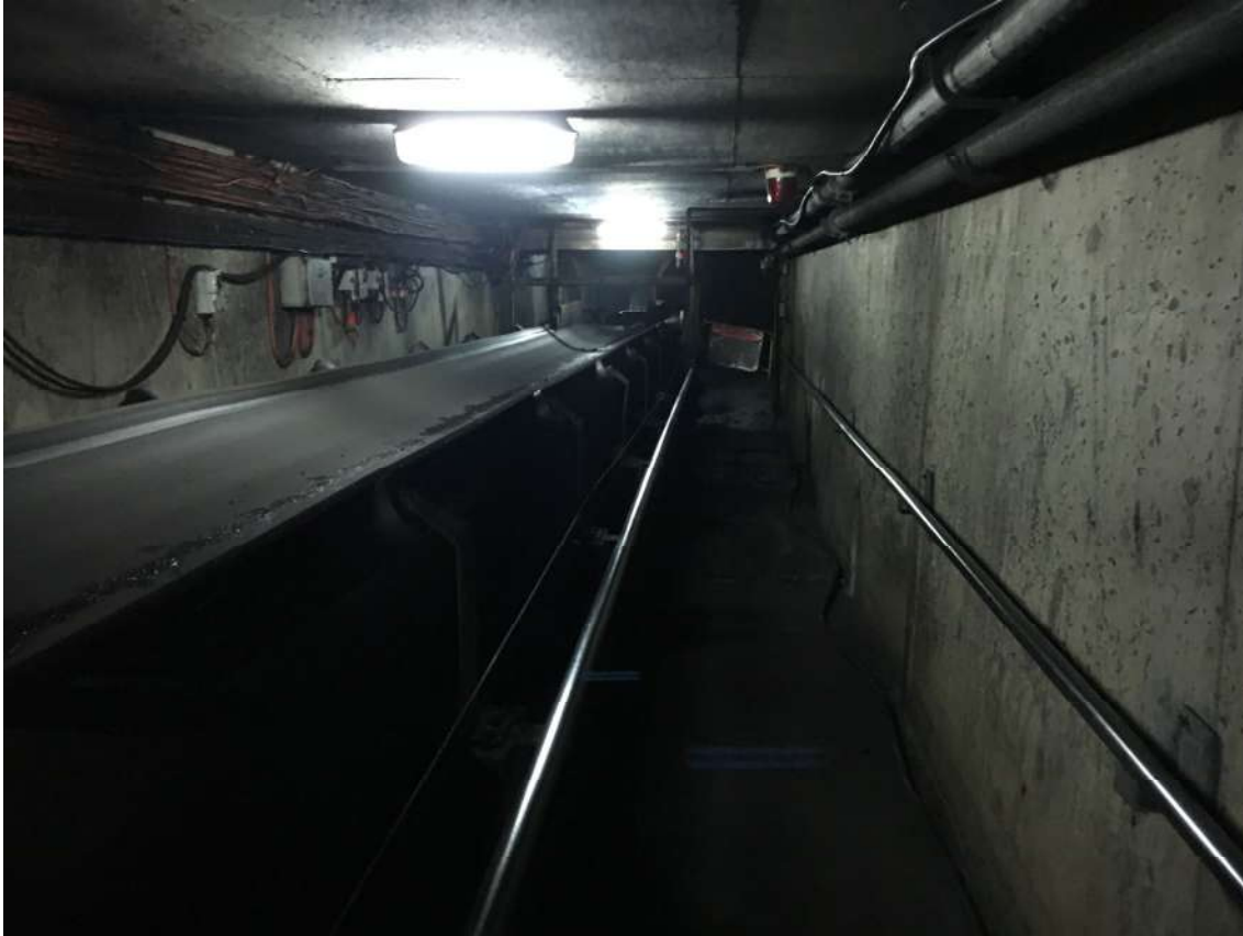
Fig. 9.5 Reclaim tunnel with Underground Conveyor 6C
