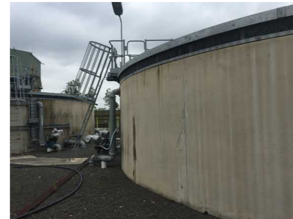
Tank 1 and Tank 2
