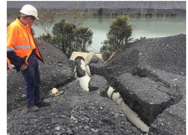
S7a scoured out inlet pipe SW corner
