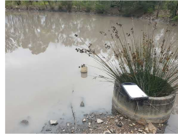
S6 Old Inundated Glory Hole (concrete) and New Glory Hole (PVC)
