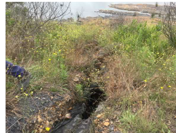
S7 Scour from Road Run-off on Western Embankment
