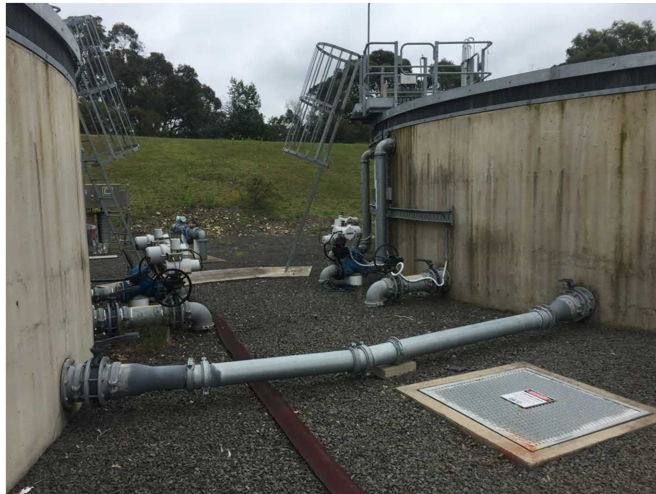
Tank 1 and Tank 2
