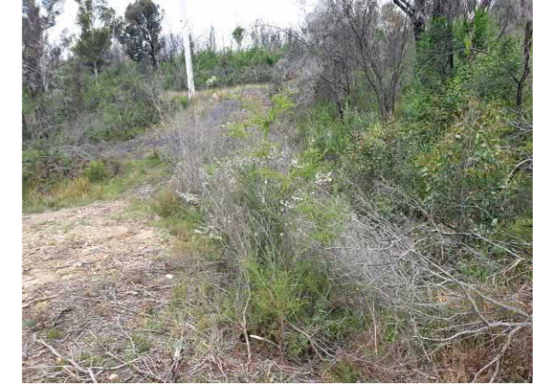
S6a Downstream Seepage of Northern Embankment
