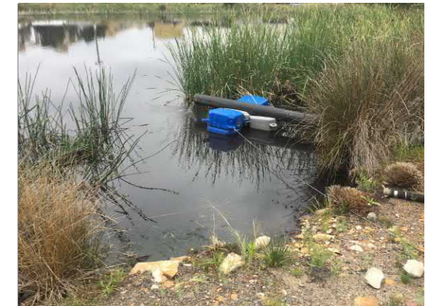
M4 WTP Feed
