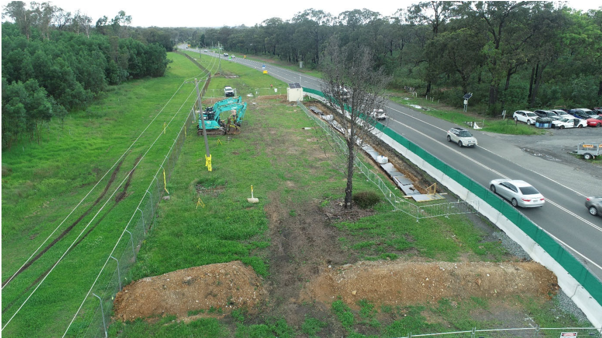
Fig. 3.31 Photograph of exposed gas main site near Pegs R47 and R48 in January 2024
