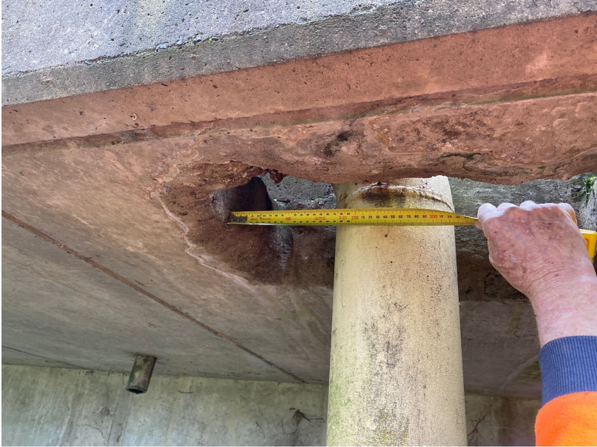
Fig. 3.39 Photograph of Jemena gas main pipe penetration for pipe bend on Remembrance Drive Bridge over the Bargo River
