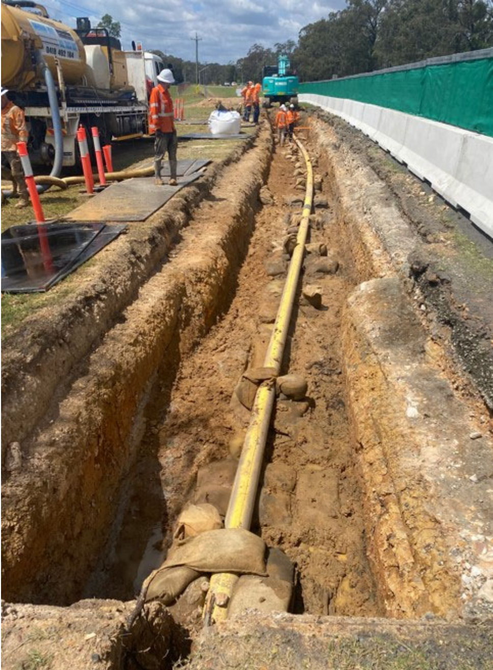
Fig. 3.30 Photograph of exposed gas main near Pegs R47 and R48 in December 2023
