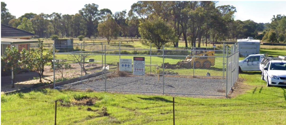
Figure 6-4: Photo of the Bargo offtake station at Hawthorne Road (Source: Google Street View).
