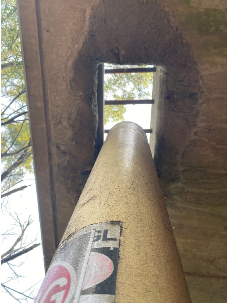
Fig. 3.38 Photograph of Jemena gas main vertical pipe bend on Remembrance Drive Bridge over the Bargo River
