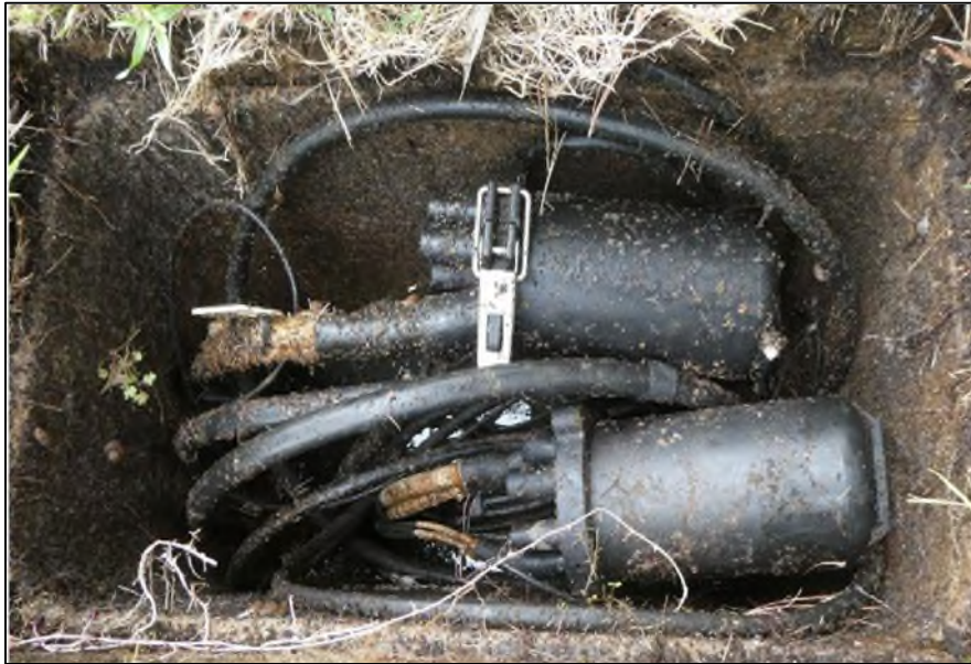
Figure 5 Typical joints in Local copper distribution cable installed along Caloola Road north side
