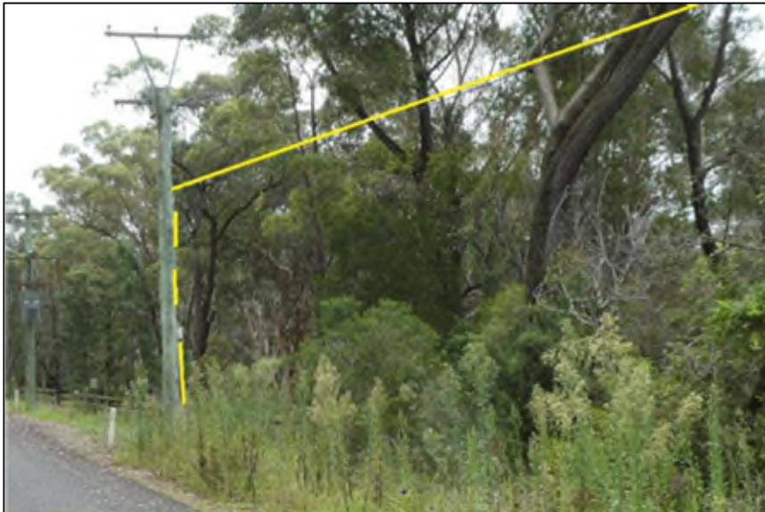
Figure 6 View west of Local aerial distribution cable in Caloola Road at the northwestern end of LW S5A
