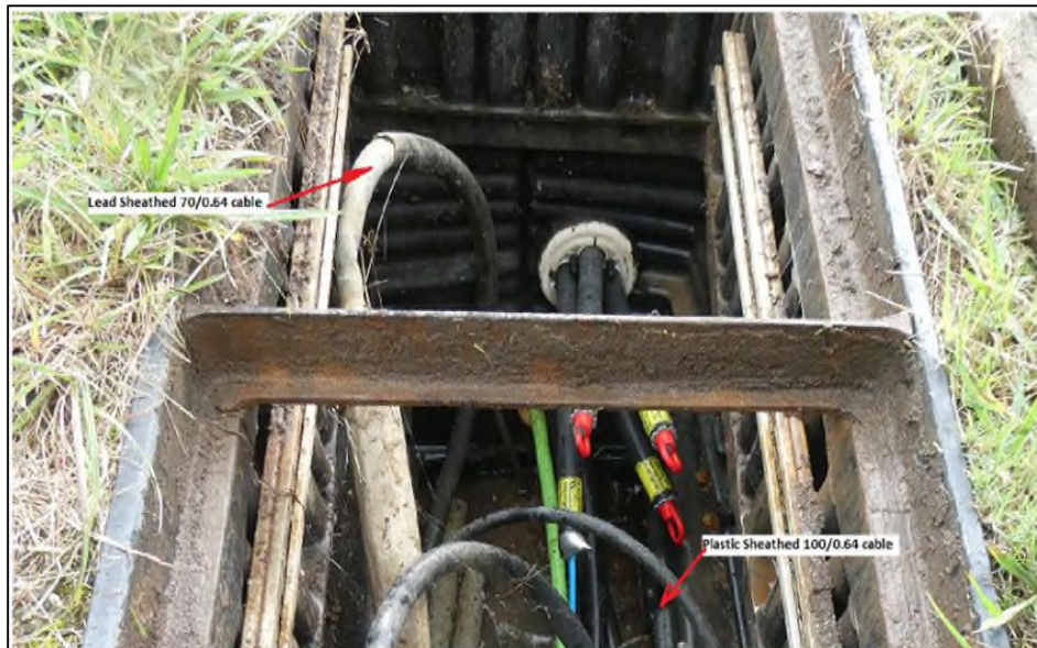
Figure 7 Typical pit showing lead and plastic sheathed cable
