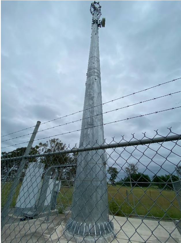
Figure 11 NBN Telecommunications Tower
