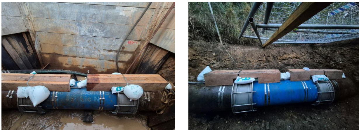
Figure 3 Gibault joints and sensors at Creek 2
